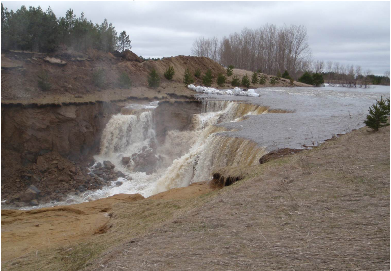
Figure 9: Severe Auxiliary Spillway Erosion
