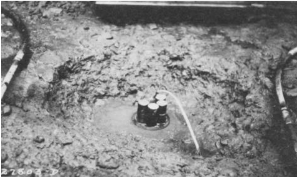
Figure C-17. Stress Meter in Place (Courtesy of the Tennessee Valley Authority).
