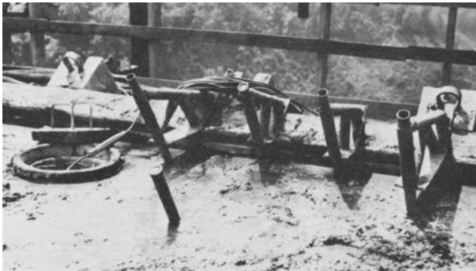
Figure C-5. Pipe Brackets for Locating Boundary Strain Meters - After Concrete is Placed (courtesy of the Tennessee Valley Authority).
