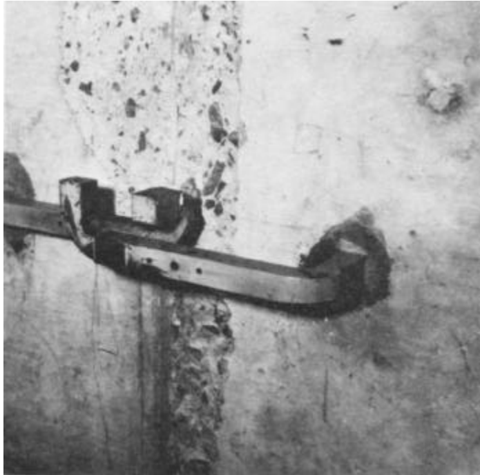
Figure 5-1. Monolith Joint Displacement Indicator. (Photo by WES)
