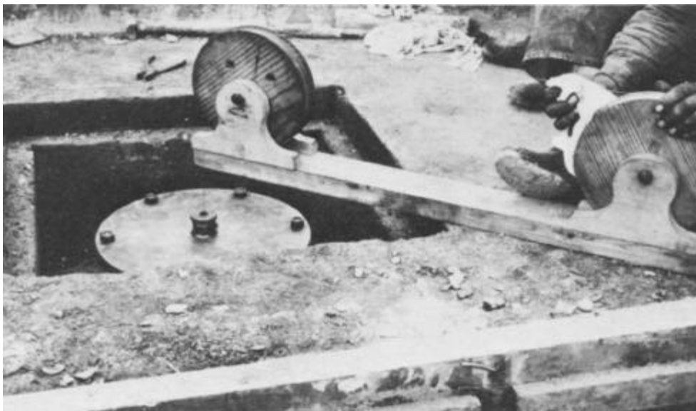
Figure 4-3. Lowering Plumb Bob Cap and Wire Through Suspension Plate (Courtesy of the Tennessee Valley Authority).
