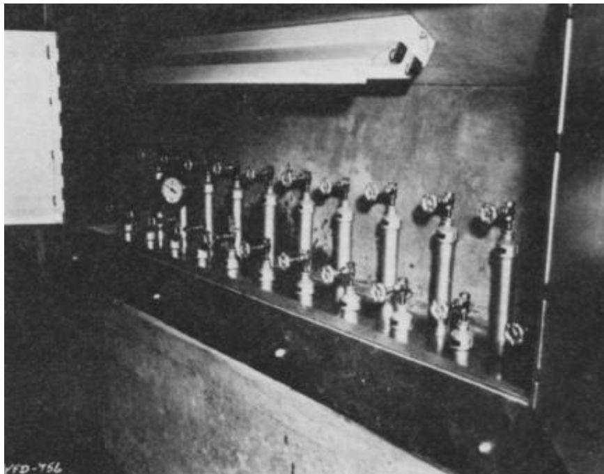
Figure 3-3. Uplift Cell Terminal Reading Station. (Photo by CE-WES)
