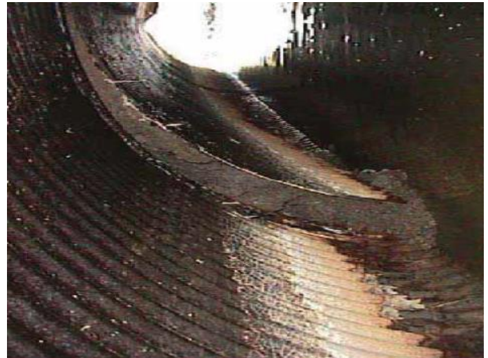
Figure 5. Joint Settlement in a CMP Conduit [2].
