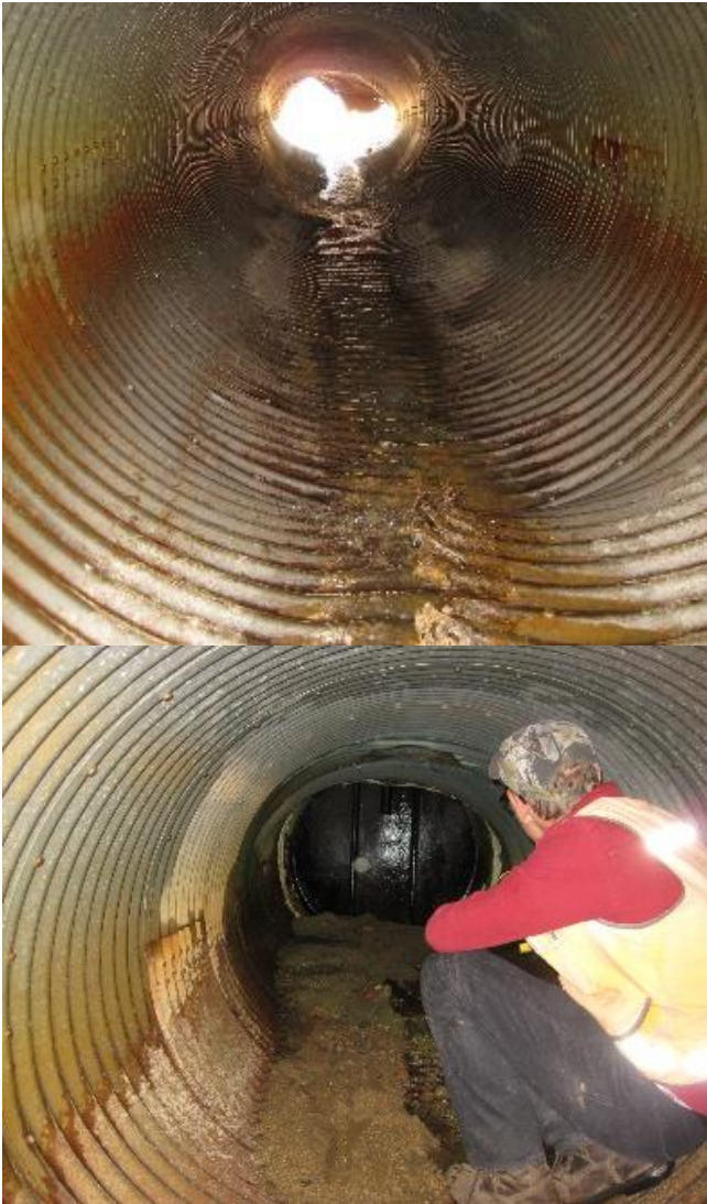
Figure 4. 48-inch CMP Failure Due to Corrosion
