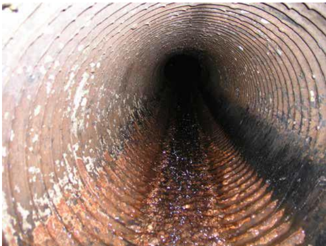
Figure 7: Minor Corrosion in a CMP Conduit [5].
