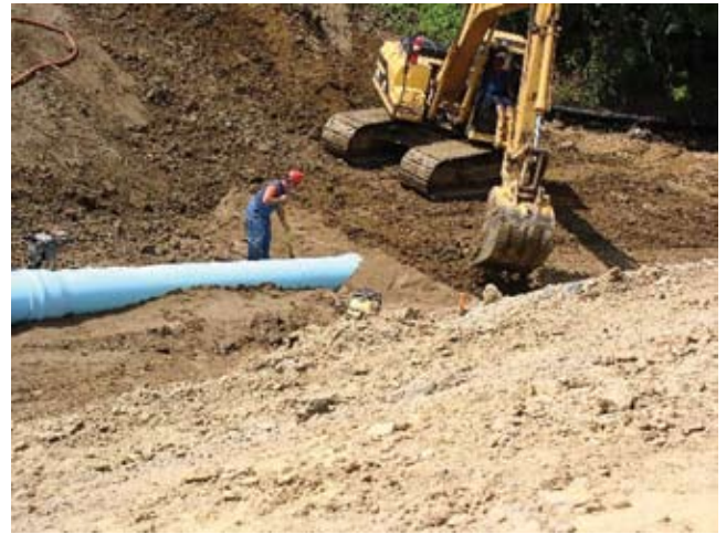
(f) Filter diaphragm being constructed above and to both sides of large diameter flexible pipe
