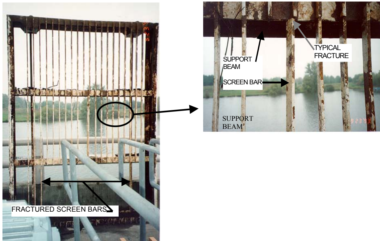
Figure 8-10. Fractured screen bars on dam intake trashrack
