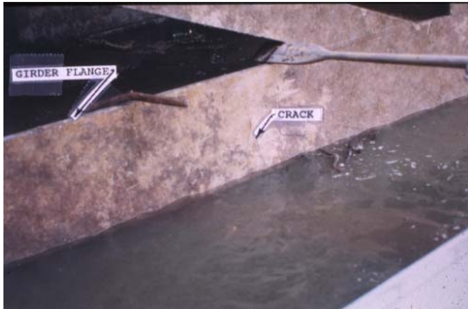
Figure 8-13. Cracked girder tension flange of a lift gate
