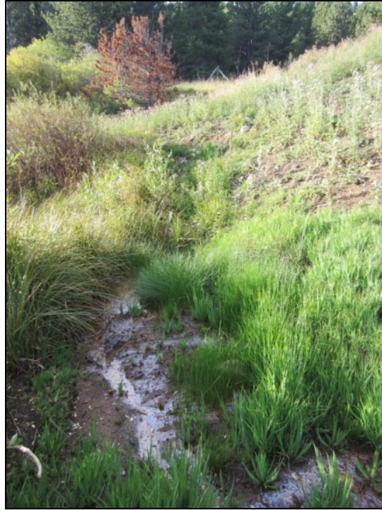
Figure 4-4: Seepage Exiting Downstream Embankment Slope (AECOM 2013)
