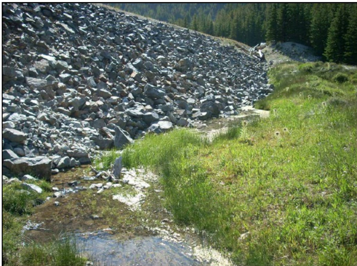
Figure 2-1: Seepage Emanating from Downstream Toe of Embankment Dam (Photo Courtesy of the DNRC)
