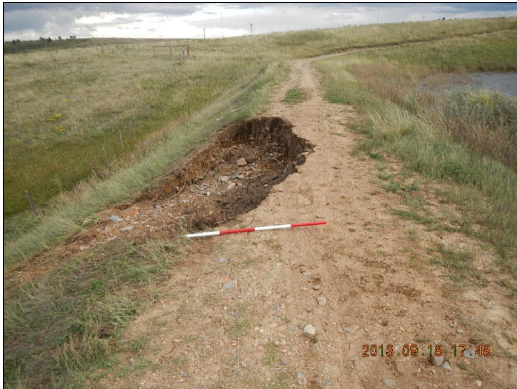
Figure 4-5: Slope Failure on Downstream Embankment Slope (AECOM 2013)
