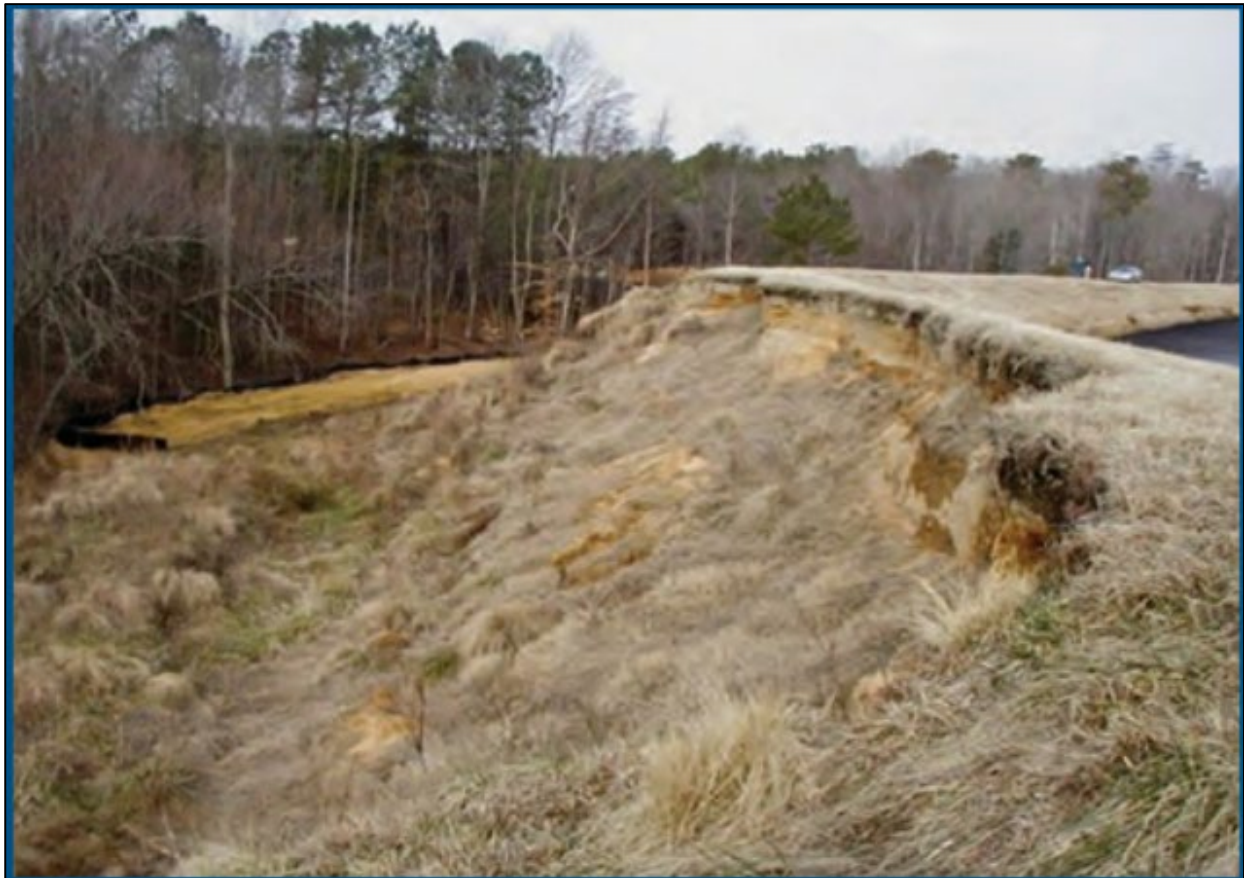
Figure 4-1: Slope Instability on Downstream Slope of Embankment Dam (FEMA 2016)
