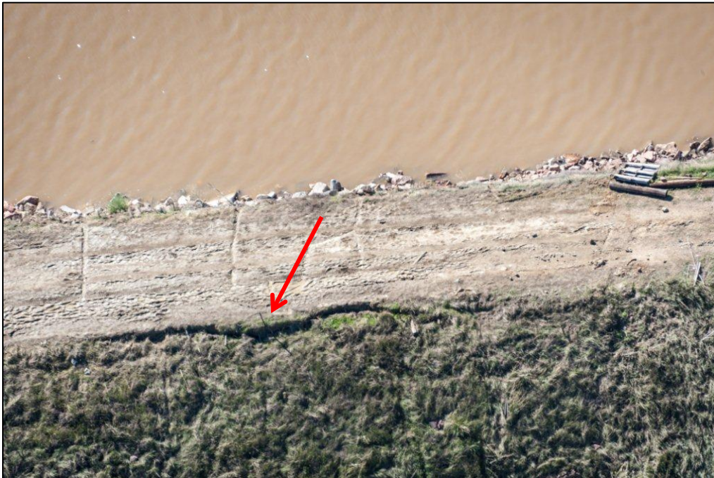
Figure 4-3: Severe Longitudinal Crack on Downstream Embankment Slope (AECOM 2013)
