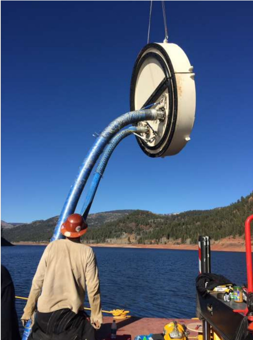
Figure 6.3.1-1. Two-piece, circular bulkhead gate being installed from a barge. Note the downstream water delivery lines extending from bottom of bulkhead gate.
