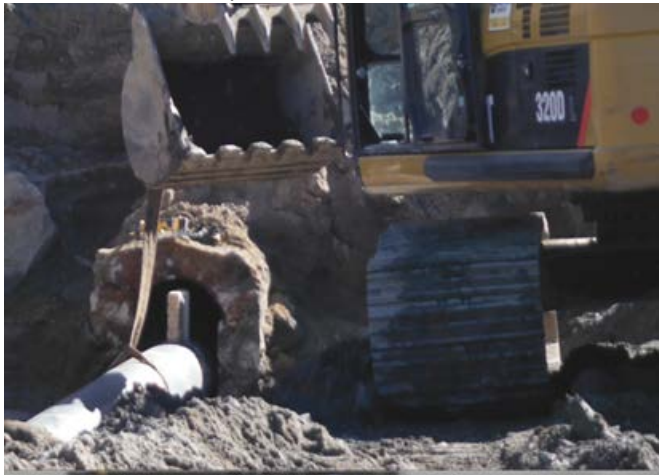
Figure 2. Conduit Sliplining with Relatively Large Annular Space Prior to Cellular Grout Placement at Estler Lake Dam
