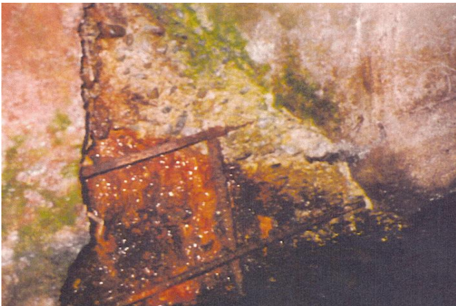
Photo 4: Spalled concrete inside a conduit. 2
