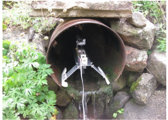
Photo 3: Manually operated CCTV sled. 3
