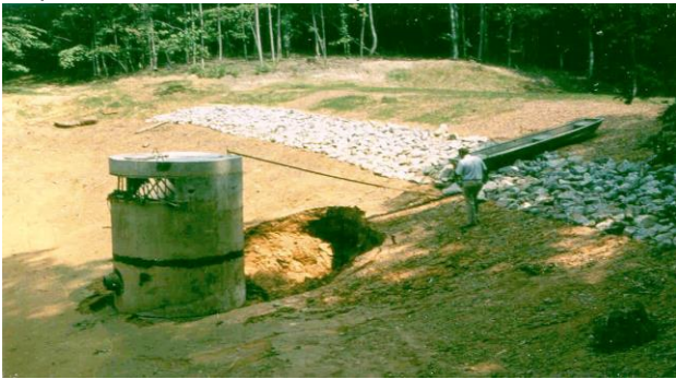
Photo 1: Sinkhole around a spillway riser 2
