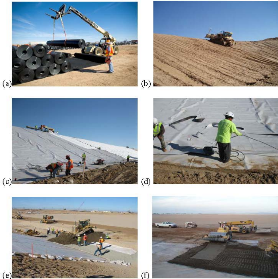
Figure 20.3.3.2-2. Warren H. Brock Reservoir lining photos: (a) handling geomembrane rolls, (b) subgrade preparation for liner placement, (c) geotextile placement over geomembrane, (d) hot wedge welding HDPE seam, (e) soil cement placement over gravel drain, and (f) soil cement protective cover over geomembrane.
