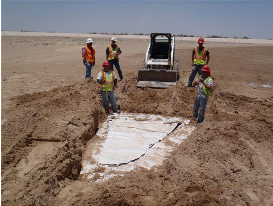
Figure 20.5.10.2-2. Large damage to geomembrane identified under a protective soil cover at Warren H. Brock Reservoir with electrical resistivity sensing.
