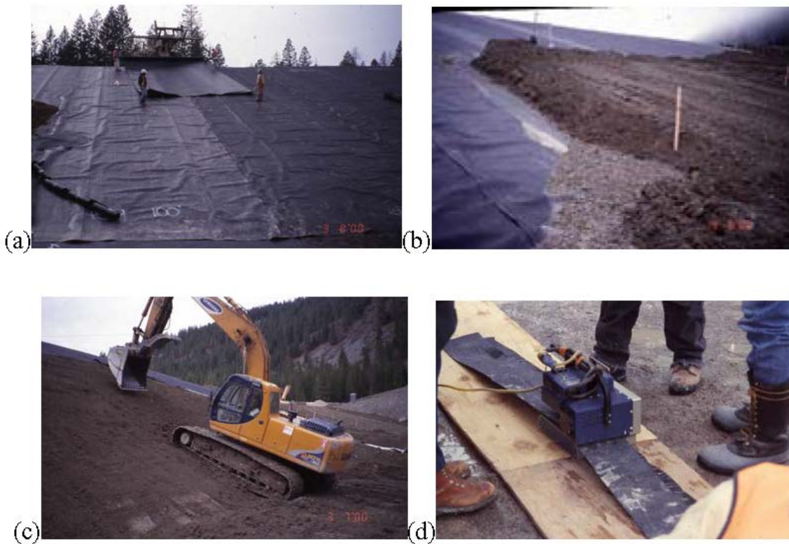
Figure 20.3.1.1-2. (a) Geomembrane deployment, (b) geomembrane and cover material, (c) geomembrane cover placement, and (d) completing pre-welds (or test welds) prior to installation of geomembrane sheets.
