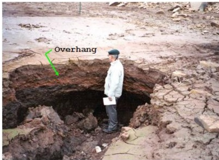
Figure 20.3.3.1-1. Sinkhole near the upstream toe of the embankment of Horsetooth Dam.
