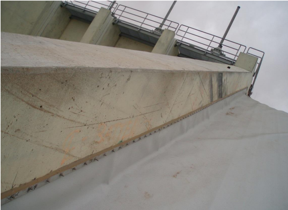
Figure 20.4.8.2-1. Connection between geomembrane and concrete structure. Stainless steel batten strip secured every 6 inches with stainless steel bolts.
