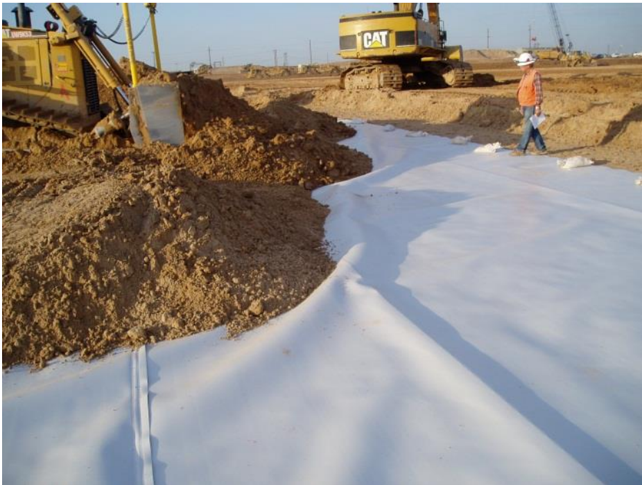
Figure 20.5.13.2-2. Development of wrinkles at the leading edge of the protective material placement.
