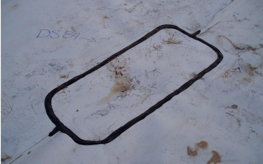
Figure 20.5.10.1-3. Destructive sample patch (Warren H. Brock Reservoir) seamed by extrusion methods (note initials and date of vacuum test on patch).
