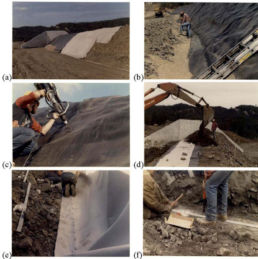
Figure 20.3.2.1-4. Pactola Dam raise construction photos: (a) geotextile and geomembrane placement, (b) key trench, (c) extrusion welding HDPE seam, (d) placement of cover material, (e) geomembrane placement atop the concrete, and (f) installing batten strip over geomembrane/concrete connection.
