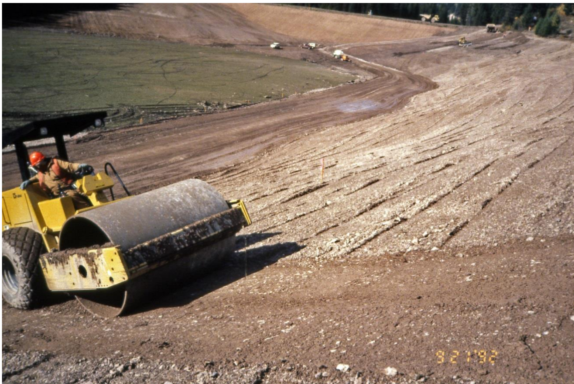
Figure 20.4.6.2-2. Final rolling of subgrade materials beneath the geomembrane liner system at Black Lake Dam, Montana (BIA).
