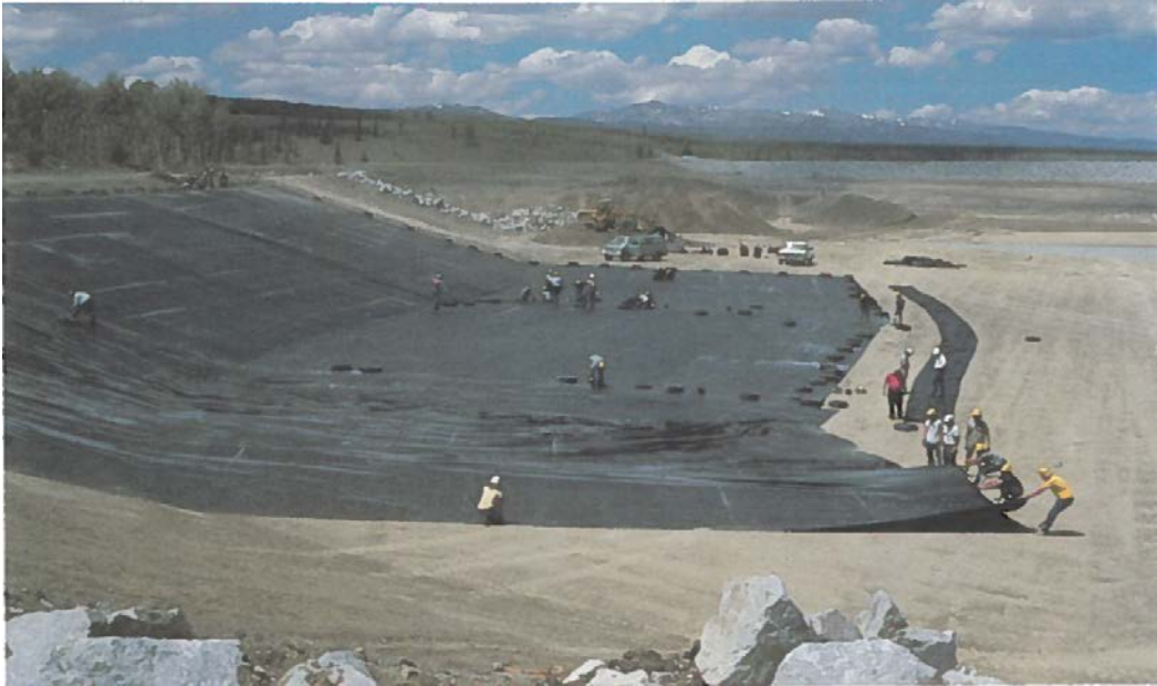
Figure 20.3.3.3-1. Installation of the Mount Elbert Forebay Reservoir geomembrane on the side slopes (note tires used as a temporary ballast during installation).
