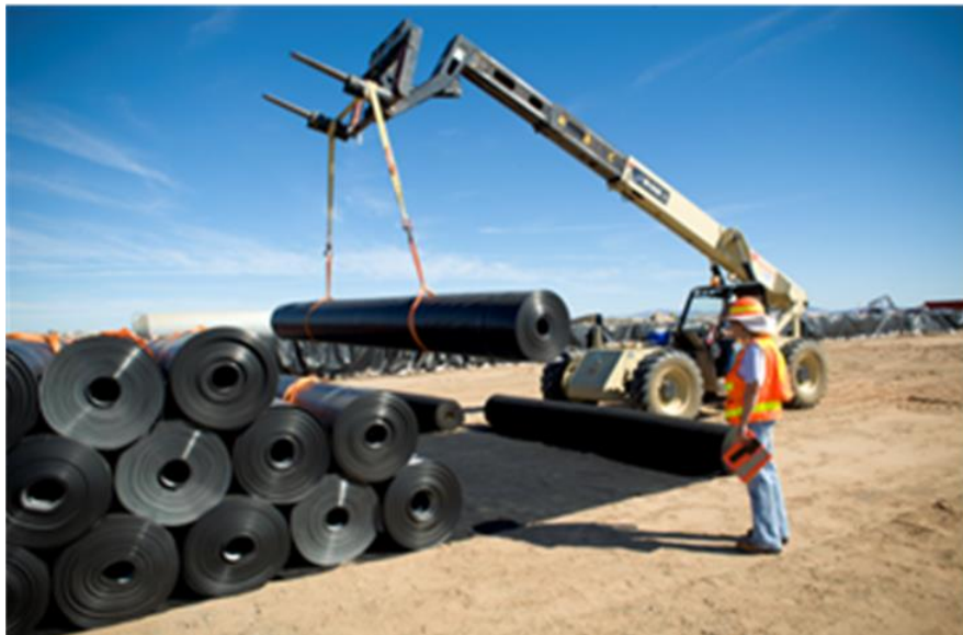
Figure 20.5.6-1. Storage of geomembrane rolls on top of geotextile to prevent damage from underlying material (note the use of nylon slings for lifting).
