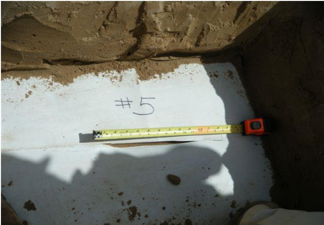
Figure 20.5.10.2-1. Small damage to geomembrane identified under a protective soil cover at Warren H. Brock Reservoir with electrical resistivity sensing.
