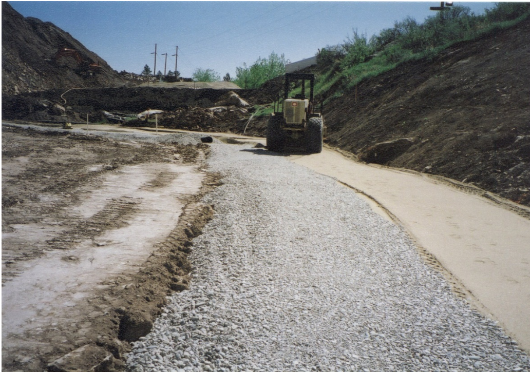
Figure 2.3.6.1-1. Placement of sand filter and gravel drain material at Spring Canyon Dam, Colorado.
