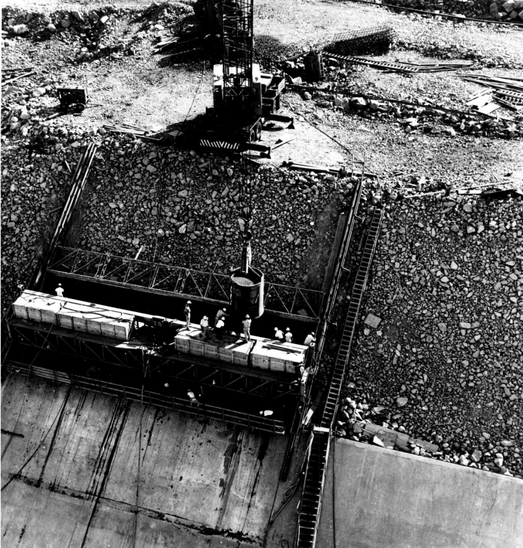
Figure 2.3.6.2-1. Placing concrete using slip forms on the upstream slope of New Exchequer Dam, California. (Tudor Engineering Company)
