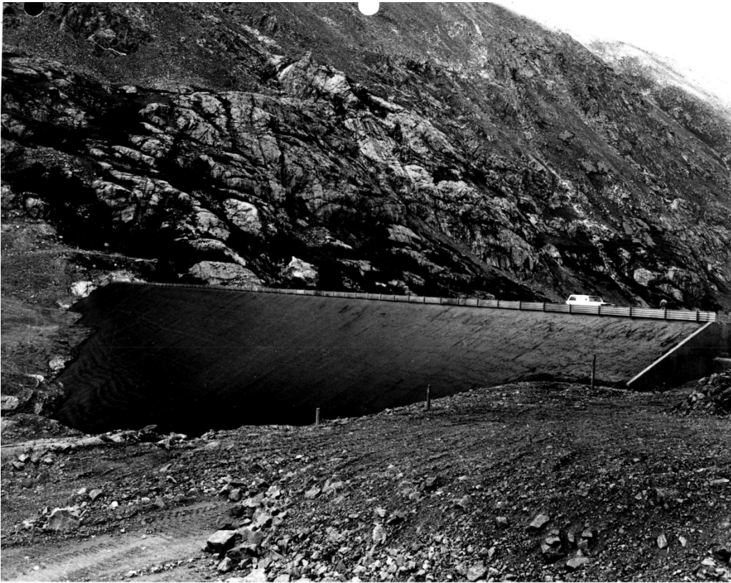
Figure 2.3.6.3-4. Completed asphaltic concrete facing at Upper Blue River Dam, Colorado. (Photo courtesy of Department of Public Utilities, Colorado Springs, Colorado.)
