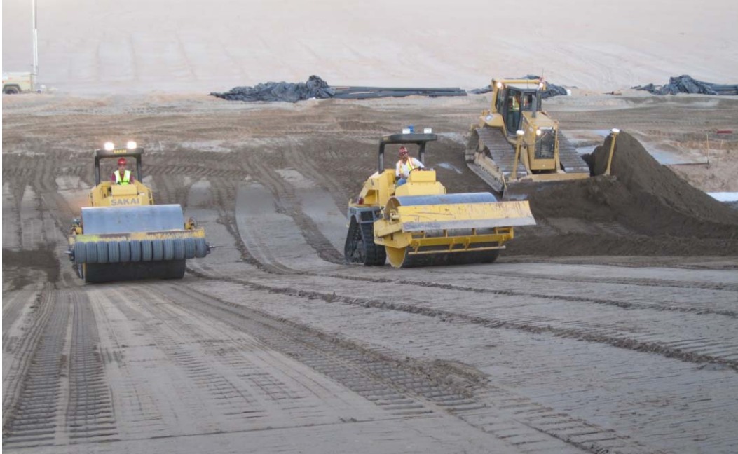
Figure 2.2.5.3.4-3. Placement of soil-cement on the interior embankment slopes of Warren H. Brock Reservoir, California, using the plating method of placement.
