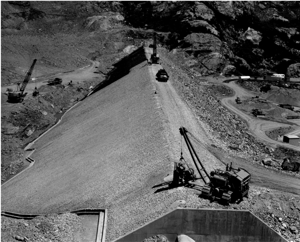
Figure 2.3.6.3-1. Completed rockfill embankment at Upper Blue River Dam, Colorado, during membrane placement. (Photo courtesy of Department of Public Utilities, Colorado Springs, Colorado.)
