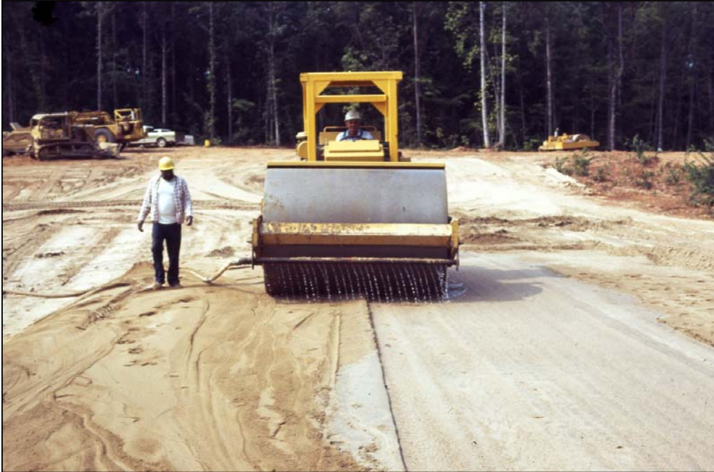
Figure 5.8.5.1.4-1. Compacting a joint between two zones by a vibratory roller. Note that the use of spray bars is no longer recommended.
