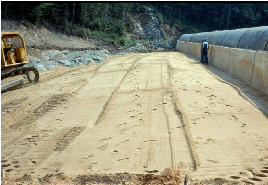
Photo 5.2.3.1-4. Filter placed over gravel blanket shown in photo 5.2.3.1-3. (Photo courtesy of NRCS, Alabama.)
