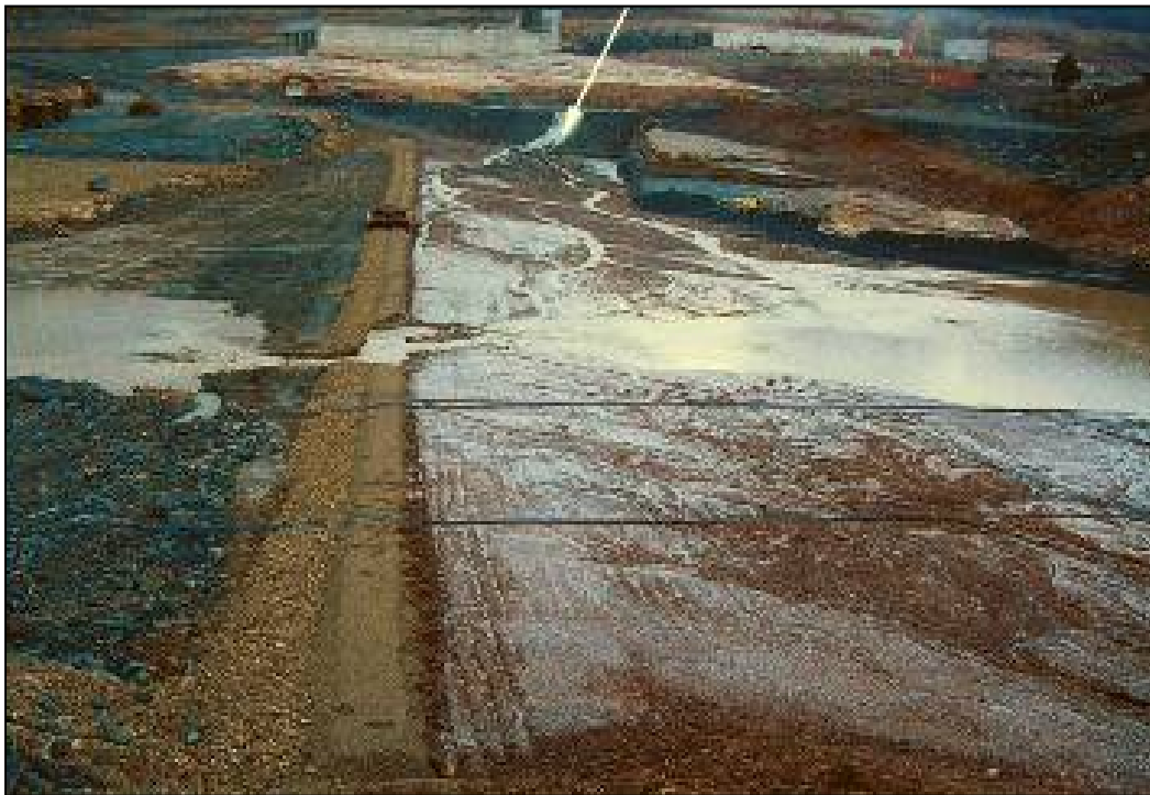
Figure 5.8.6.1.1-1. Surface water contamination of a chimney filter.
