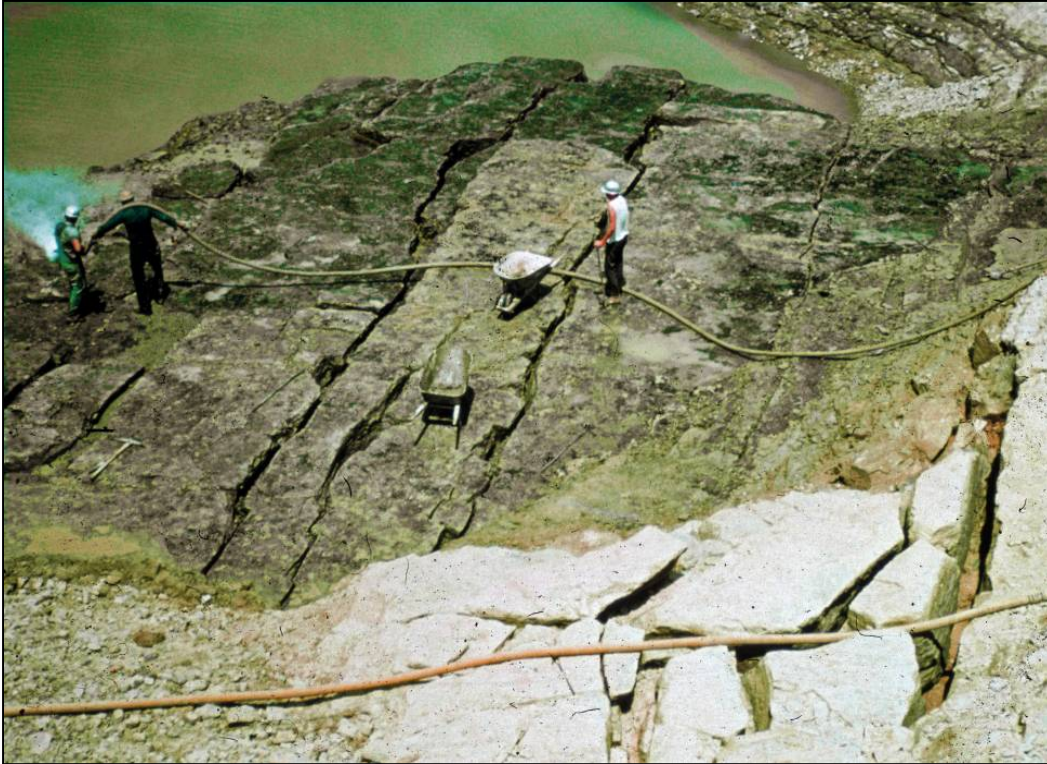
Photo 5.2.3.1-1. Pressure washing joints and fractures in bedrock prior to dental grouting and covering with a blanket under the downstream shell of a dam. (Photo courtesy of NRCS.)
