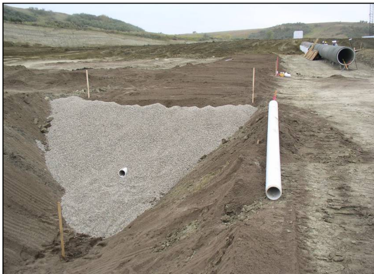
Photo 5.2.3.2.1-2. Trapezoidal foundation trench drain at toe of embankment. Coarse inner filter (envelope) surrounds perforated collector pipe, and the fine filter provides filter compatibility with foundation soils.
