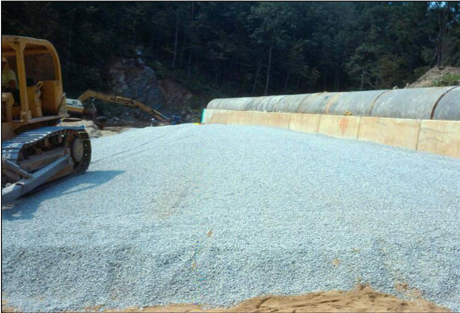
Photo 5.2.3.1-3. Gravel blanket being placed over filter shown in photo 5.2.3.1-2. (Photo courtesy of NRCS, Alabama.)
