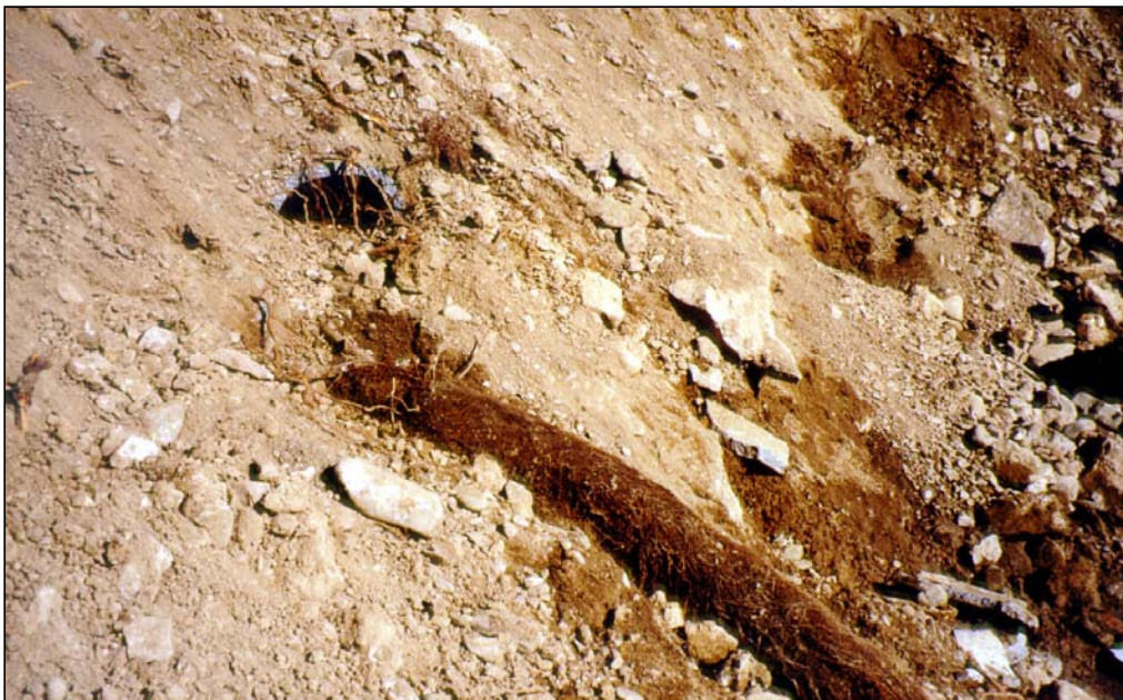
Photo 5.2.3.5-4. During modification of a dam, this toe drain pipe was exposed during excavation. The pipe was completely clogged with the root ball shown in the foreground. It was noted that a tree was growing over the toe drain, and the drain was probably a water source in this arid region of central Oregon.
