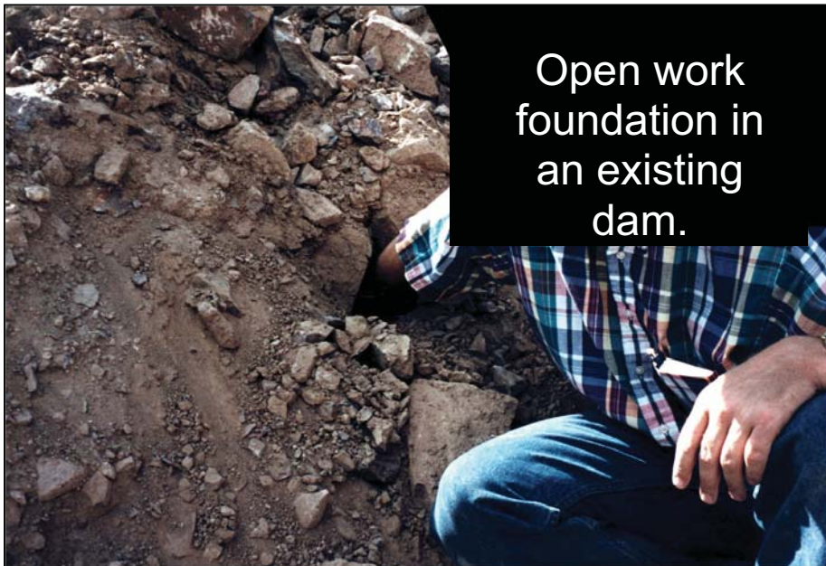
Photo 5.2.3.1-5.—Open work present in the right abutment foundation of Ochoco Dam. The abutment consists of landslide debris.
