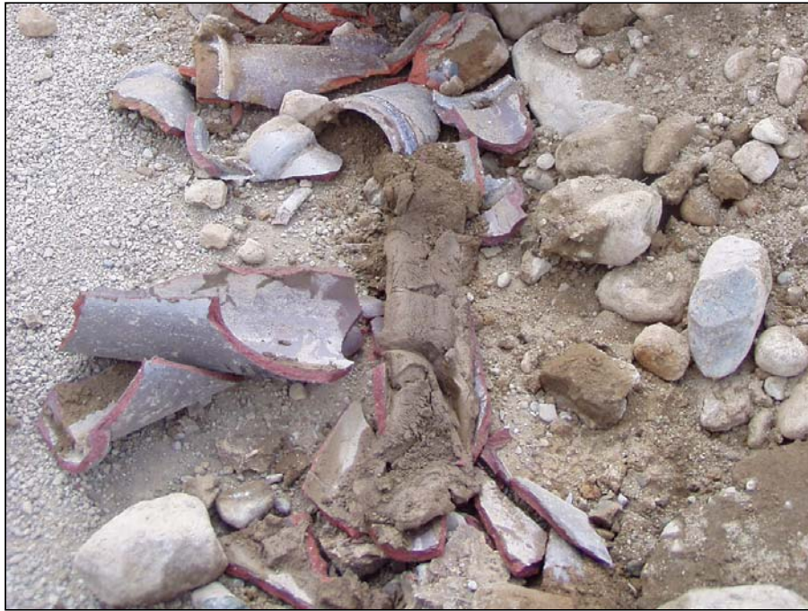
Photo 5.2.3.5-3. Clay tile pipe from 1916 as it was exposed during excavation. Note that the pipe was completely clogged with silt and sand.
