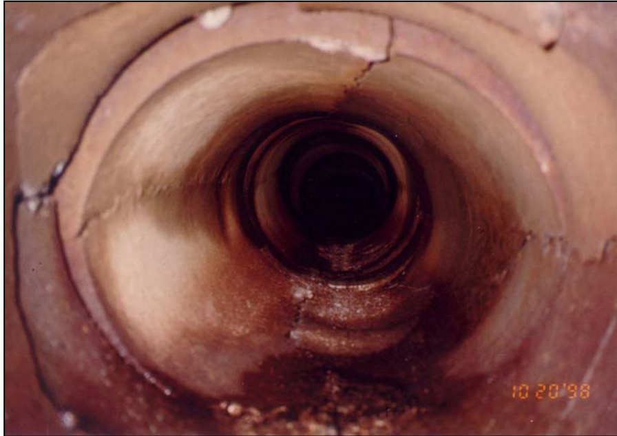
Photo 5.2.3.5-2. Interior view of a reinforced concrete pipe from the 1950s. Note that the pipe is overstressed, and cracks have formed at the crown and spring line. The pipe has also deformed to an oval shape. In the foreground, a joint can be seen and sand that passed through the joint.
