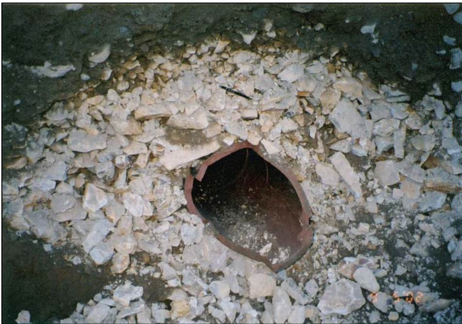
Photo 5.2.3.5-1. Clay tile pipe surrounded by gravel-size material. Note mechanical pencil for scale. Surrounding the gravel is a mixture of silt and sand backfill that does not meet filter criteria for the gravel. Seepage enters the pipe through joints between pipe segments. The silt and sand can erode through the gravel backfill and enter the pipe through the joints.
