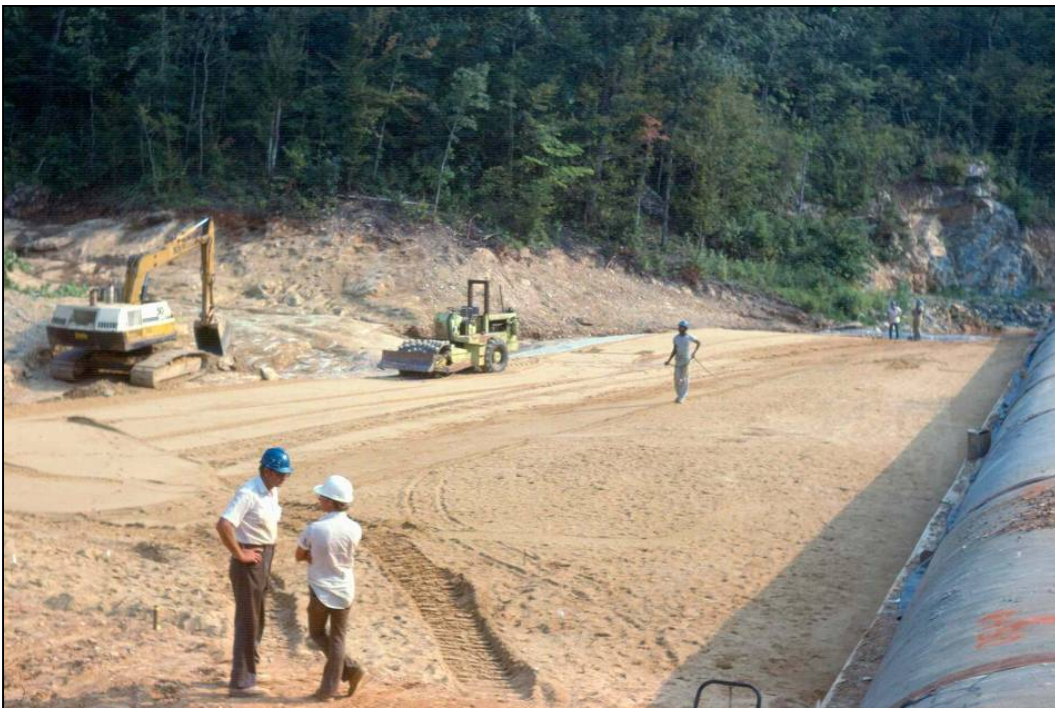
Photo 5.2.3.1-2. Filter being placed on the bedrock surface under the downstream shell of an embankment. View is toward downstream toe. Conduit is to the right of the photograph. Exposed bedrock not yet covered is in the background behind trackhoe. (Photo courtesy of NRCS, Alabama.)
