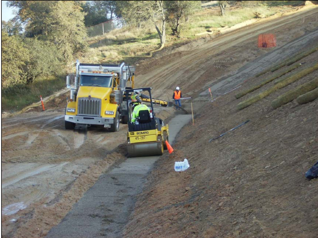
Figure 5.8.2.6-1. Truck conveyor delivering filter sand for the addition of a 4-foot-wide chimney filter to an existing embankment. Note that the material is uniformly placed from the conveyor, and no leveling is required. Dynamic compaction is provided by the roller shown in the foreground.
