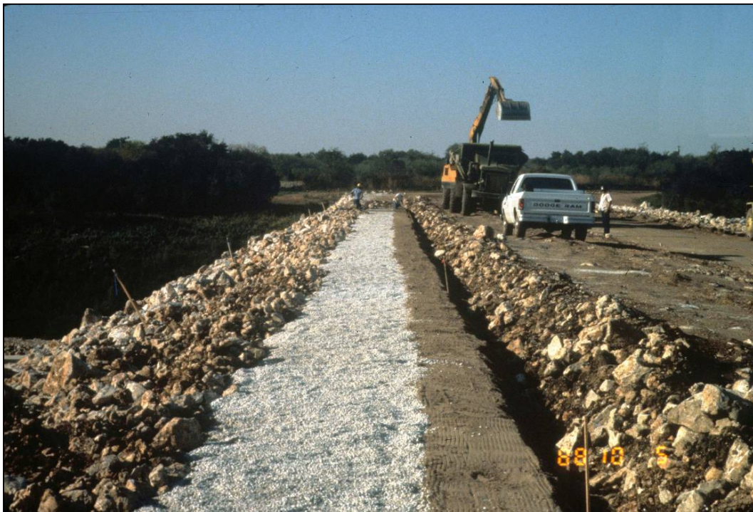
Photo 5.2.2.3-1. Two-stage chimney being constructed in zoned dam by concurrent method of construction.
