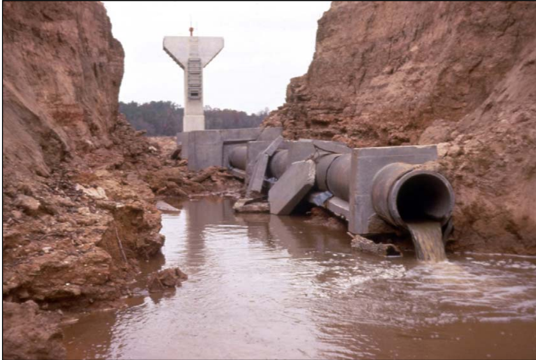
Photo 5.2.2.4.1-1. Embankment dam breached after piping along the conduit. The view is upstream. Note precast concrete pipe placed on a concrete cradle that did not completely fill the haunch and the use of seepage collars. Note that the cradle only partially fills the haunch.
