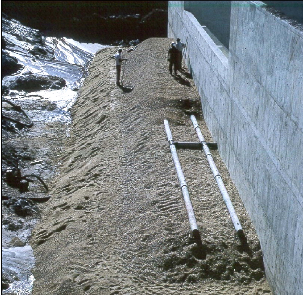
Photo 5.2.2.4.3-1. Filter and drainage zones to provide pressure relief and drainage of backfill next to training wall for a spillway chute. (Photo courtesy of NRCS, Texas.)
