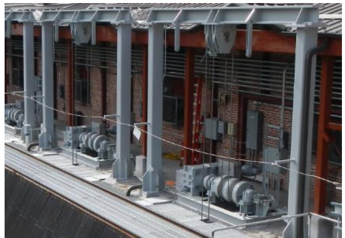
Photo 1: Wire Rope Hoisting Systems for Fixed Wheel Gates
