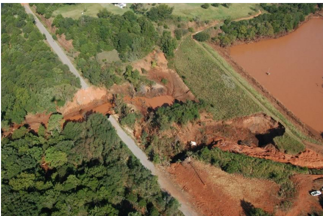
Figure 6 – Sugar Creek L-44 Spillway and Dam Erosion
