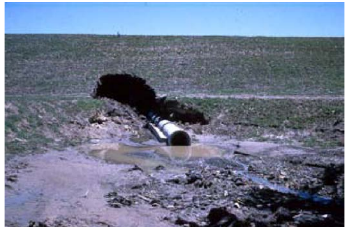
Photo 4: Piping failure along outlet conduit
