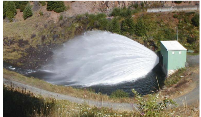
Photo 5: A cone valve dissipates energy downstream of an outlet works
