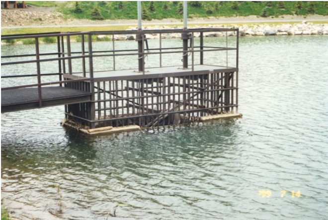
Photo 2: Trash racks surrounding an intake structure
