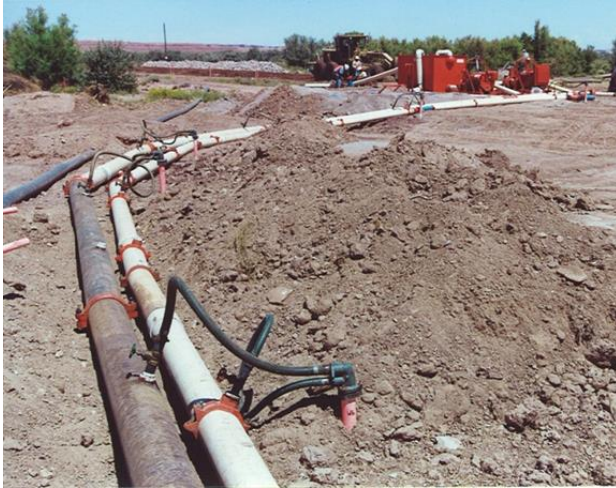
(a) High pressure and extraction pumps.
