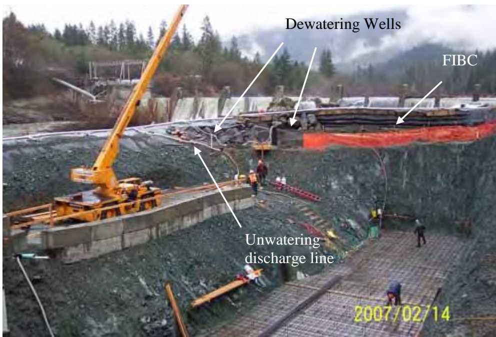
Figure 21.8.9-1. Excavation dewatering and unwatering behind soldier pile and sandbag (FIBC) cofferdam on the Rogue River, Oregon (Savage Rapids Dam Removal and Replacement Pumping Facilities, Grant Pass Project, Oregon, photo by Reclamation Yakima Office staff).
