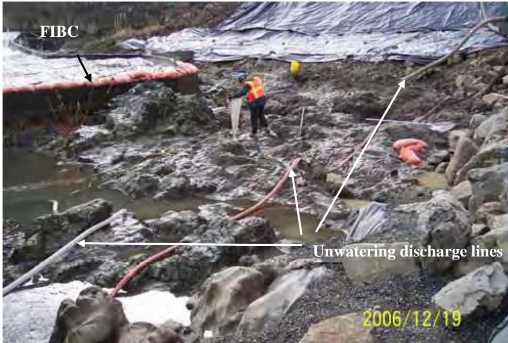
Figure 21.8.6.4-1. Unwatering behind a sandbag cofferdam on the Rogue River, Oregon. Cofferdam consists of flexible intermediate bulk containers (FIBC) (also called big bags, bulk bags, or jumbo bags) filled with local sands and soils. Open pumping is removing standing water in a number of pools of various sizes and depths (Savage Rapids Dam Removal and Replacement Pumping Facilities, Grant Pass Project, Oregon, photo by Reclamation Yakima Office staff).
