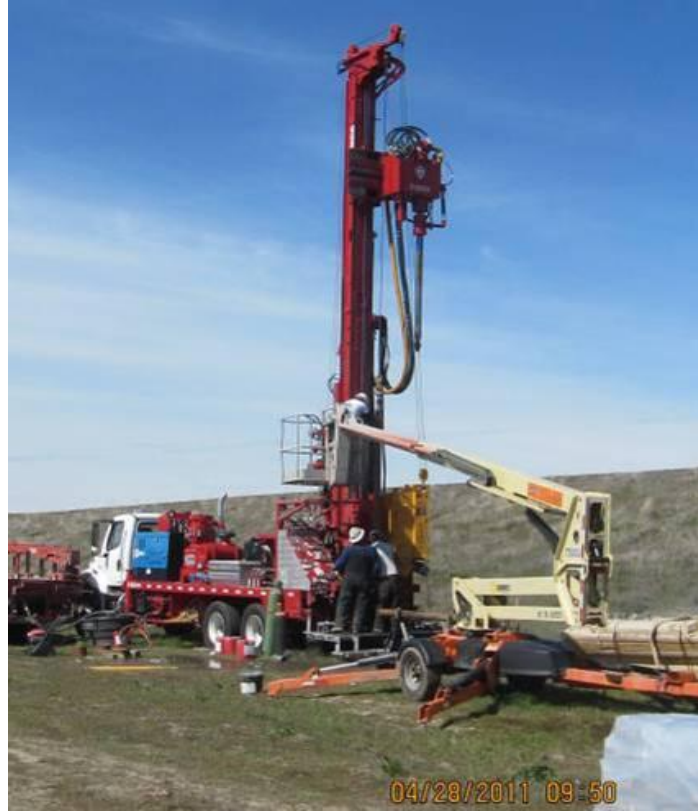
Figure 21.9.2-5. Upper Colorado Region drill crew's Gus Pech 3000 CHR top head rotary rig; 30,000 torque, 32,600 pounds pull back (photo by Scott Jensen, Reclamation's Upper Colorado drill crew, A.V. Watkins Dam, 2011).
