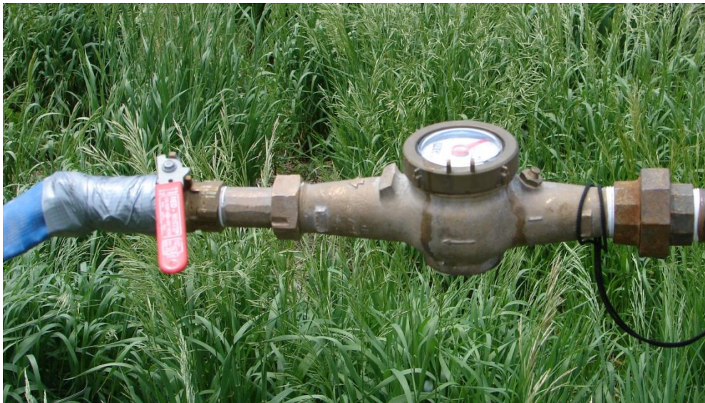
Figure 21.8.10-3. Totalizer in-line flow meter installed in a straight section of discharge line (closeup view). Straight sections of pipe are required both upstream and downstream of the flow meter to ensure non-turbulent flow through the meter for accurate readings. Upstream length was 2 feet, downstream length was 1 foot because of the low sustained discharge rate obtained during this test. Note the butterfly valve at the end of the pipe section used to control discharge rates (Red Willow Dam, Nebraska, photo by W. Robert Talbot).
