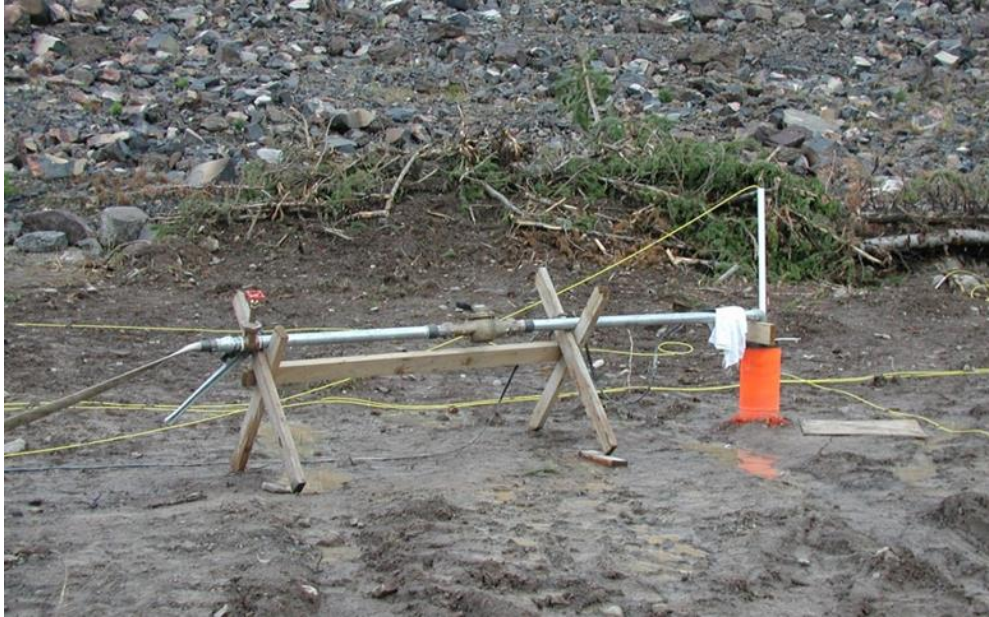
Figure 21.8.10-2. Totalizer in-line flow meter installed in a straight section of discharge line. Straight sections of pipe are required both upstream and downstream of the flow meter to ensure non-turbulent flow through the meter for accurate readings. Required lengths of straight sections of pipe will vary with meter size and design (Grassy Lakes Dam, Wyoming, photo by W. Robert Talbot).
