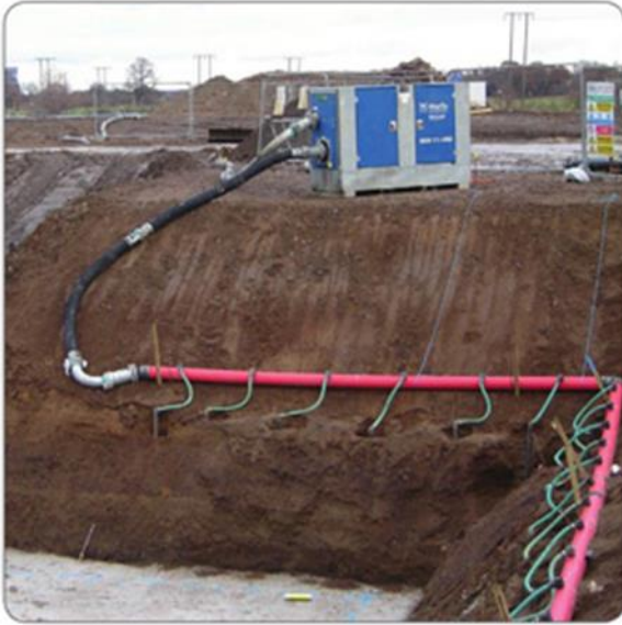
Figure 21.8.5.2-1. Single stage (one layer) well-point system (reprinted with permission of Shortflo dewatering system, Groundforce, UK).
