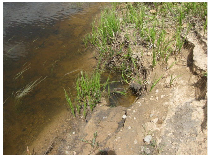
Photo 1: Example of small depression that may go unnoticed (Young Creek Dam)
