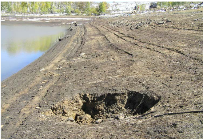
Photo 3: Sinkhole on upstream embankment (Paxton Dam)
