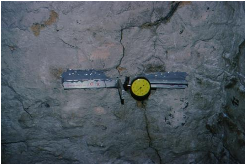
Figure 69. A dial gauge used to monitor crack movement.
