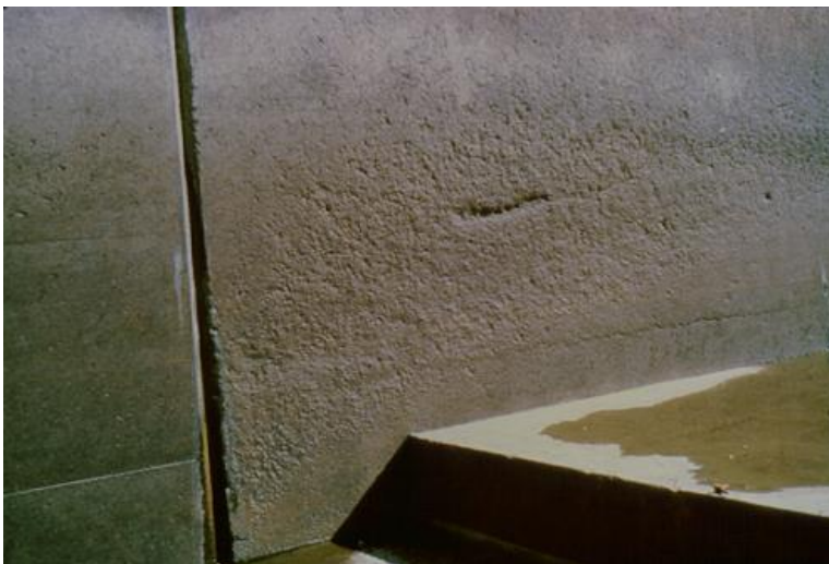
Figure 61. The early stages of concrete erosion from ebrasion and possible cavitation. Subsequent damage may lead to further cavitation damage.
