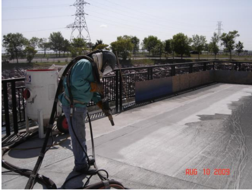
Figure 26. Sand blasting a concrete deck prior to application of a healer-sealer (Sealers and Coatings).
