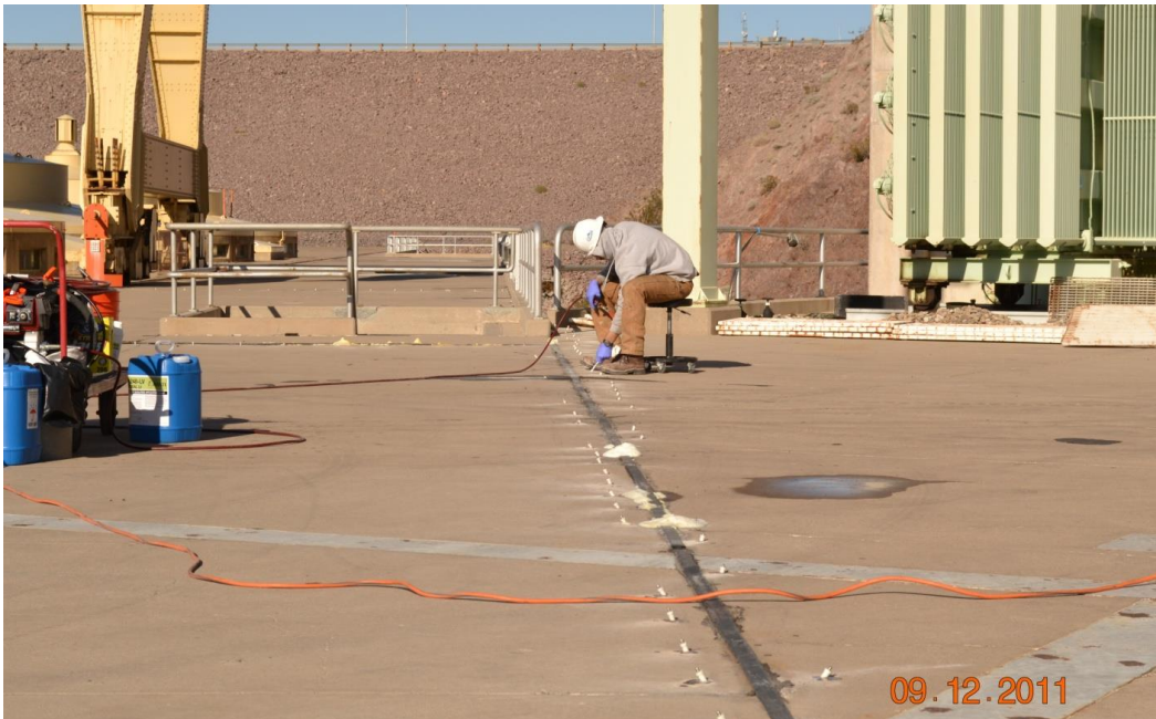
Figure 127. Grouting is progressing from one end of the leaking expansion joint to the other. The presence of foam indicates that the joint is full of grout. The grout is contained by packing the joint with jute from below, the joint sealant at the top of the joint, and the zerk fittings on the ports.
