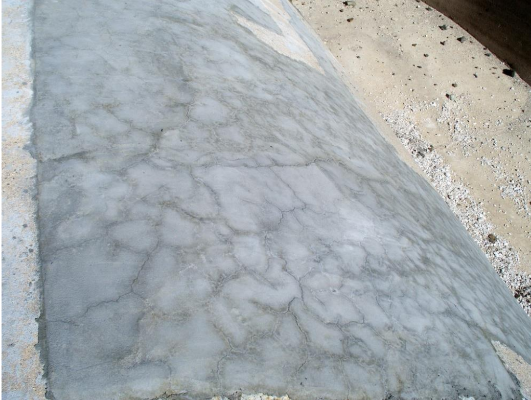
Figure 99. Extensive cracking in a packaged thin repair mortar applied to a spillway crest. Unfortunately, this occurs too often for thin repair mortars.
