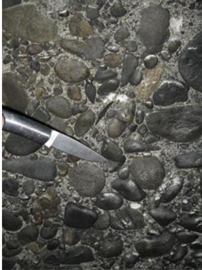
Figure 56. Abrasion-erosion damage from flowing water with small abrasive particles showing a polished surface.
