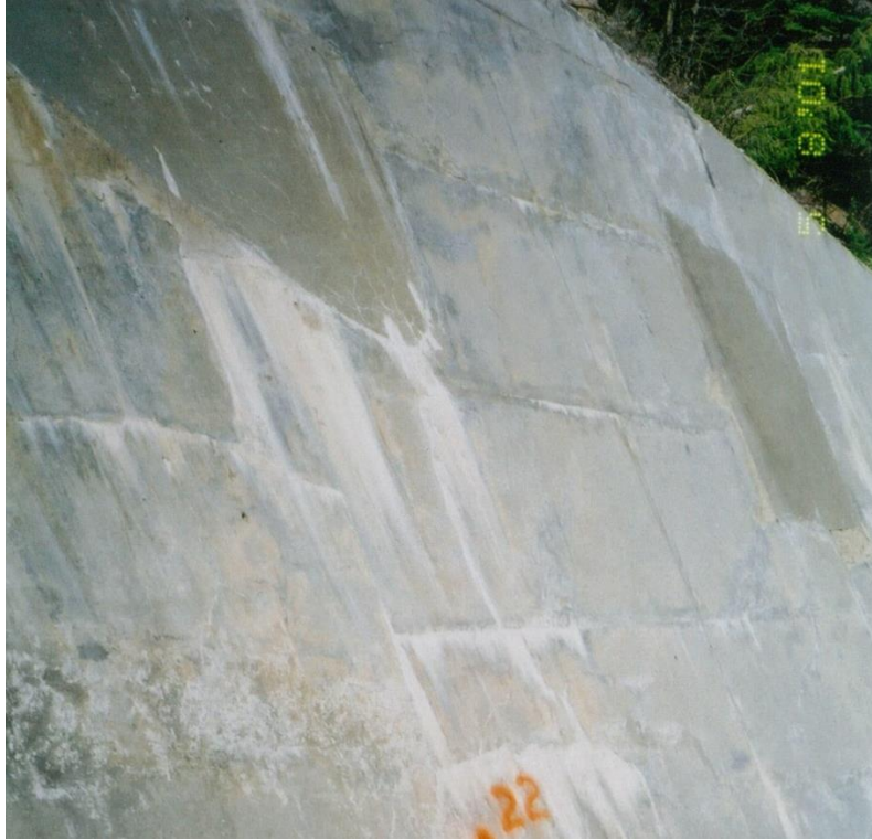
Figure 84. Insufficiently thick repairs on a spillway wall made with concrete subject to freeze-thaw deterioration resulted in failure of the repair and additional damage to the surrounding concrete.
