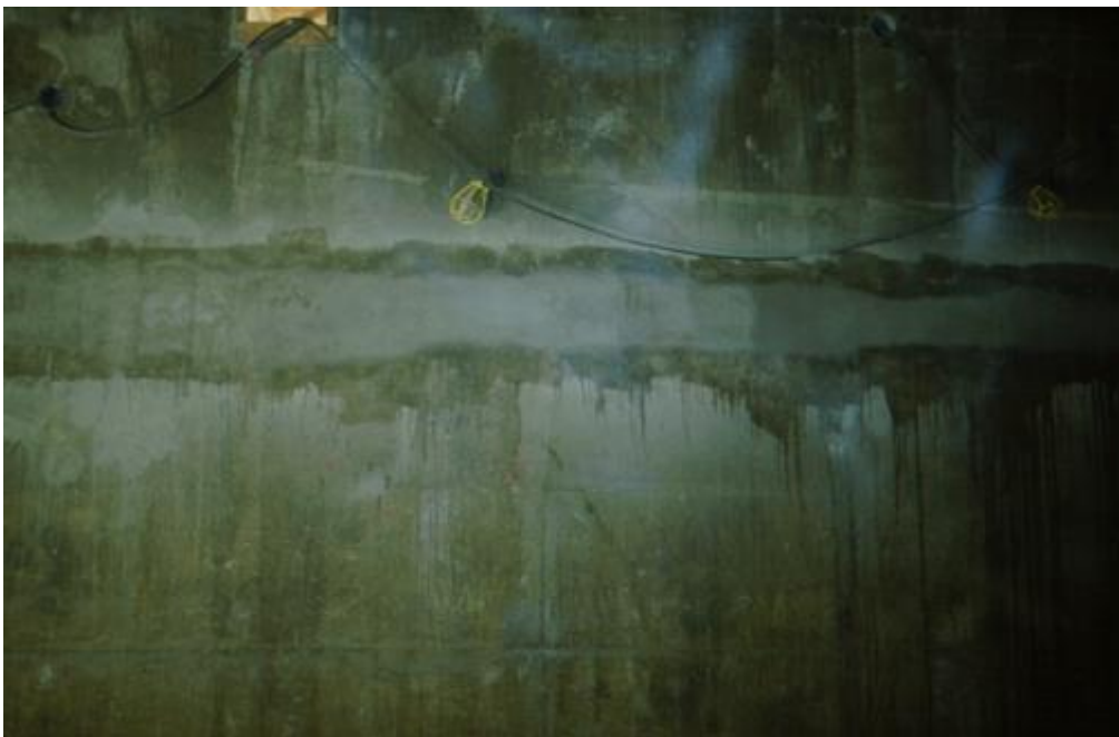
Figure 86. Portland cement mortar repairs made to a shallow defect. Note how it differs in color from the parent concrete.
