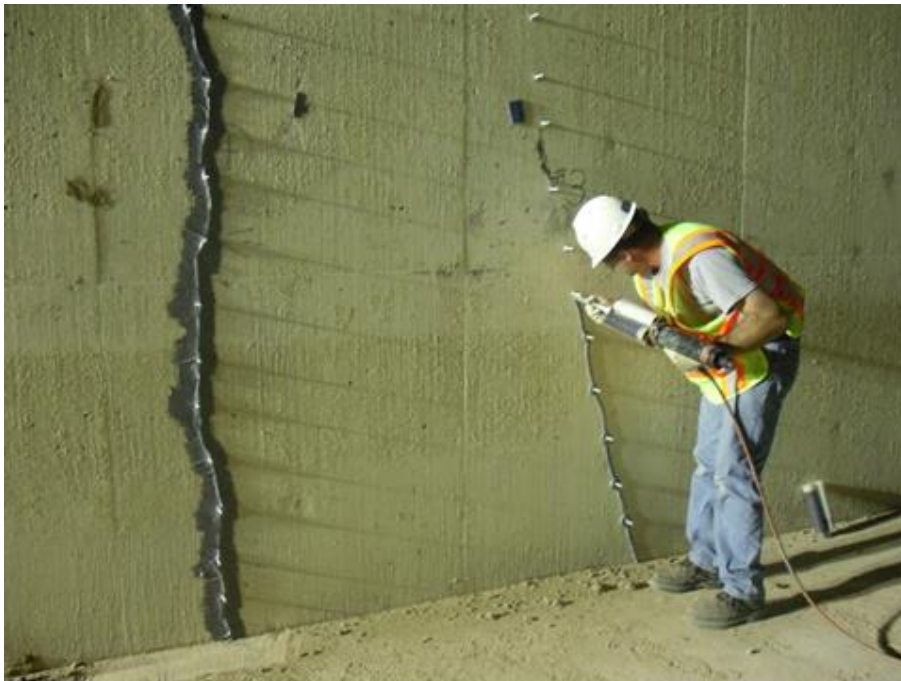
Figure 114. Sealing the crack opening for epoxy resin injection after attaching the injection ports.
