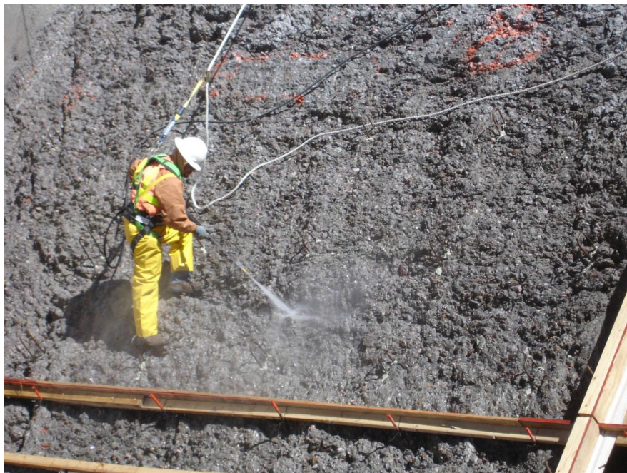
Figure 16. After beginning concrete removal, the extent of damage was much worse than originally believed. Concrete was easily removed due to extensive deterioration.
