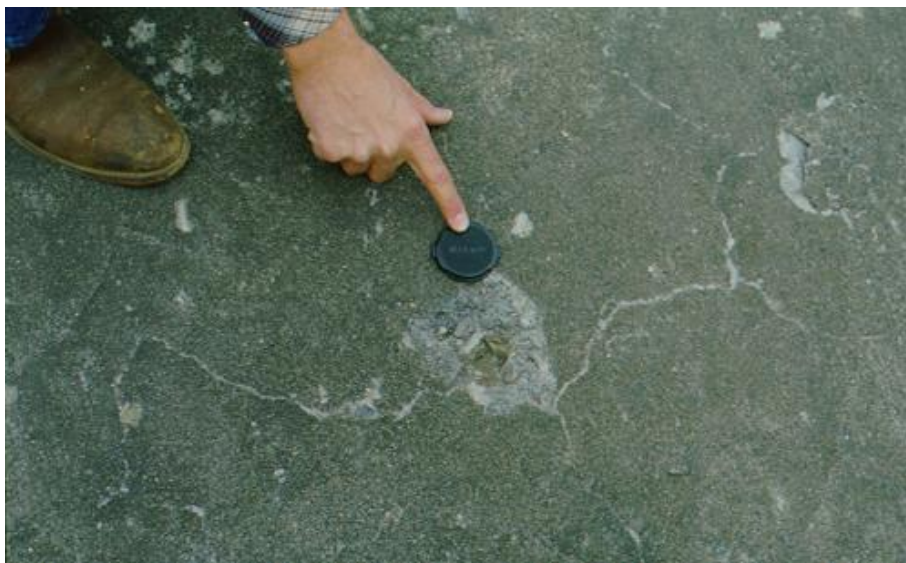
Figure 11. Damage from absorptive aggregates.
