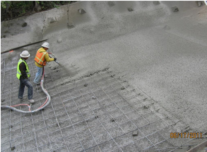
Figure 104. Using shotcrete to repair a spillway floor. Shotcrete was used here because of the remoteness of the site.
