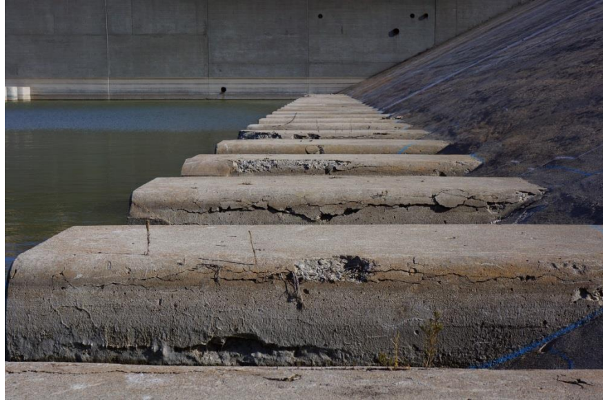
Figure 12. Damage from absorptive aggregates deteriorating from freezing and thawing weather that extends several inches into the concrete.
