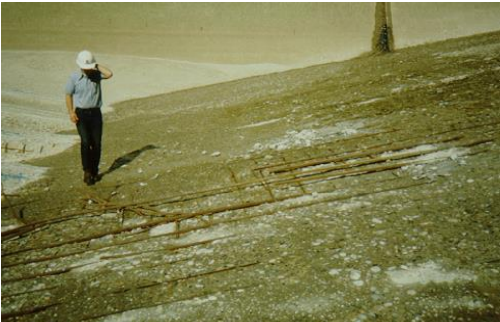
Figure 13. Damage that appears serious, but because of the characteristics of the spillway, repairs are not needed immediately.
