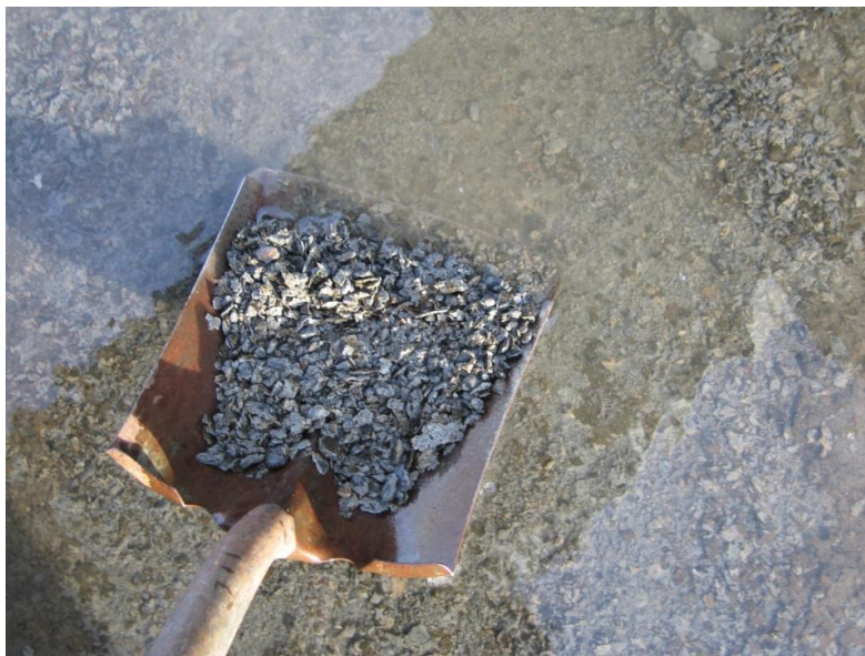
Figure 43. Salt scaling that resulted when water containing deicing salts froze on poor quality concrete surfaces.
