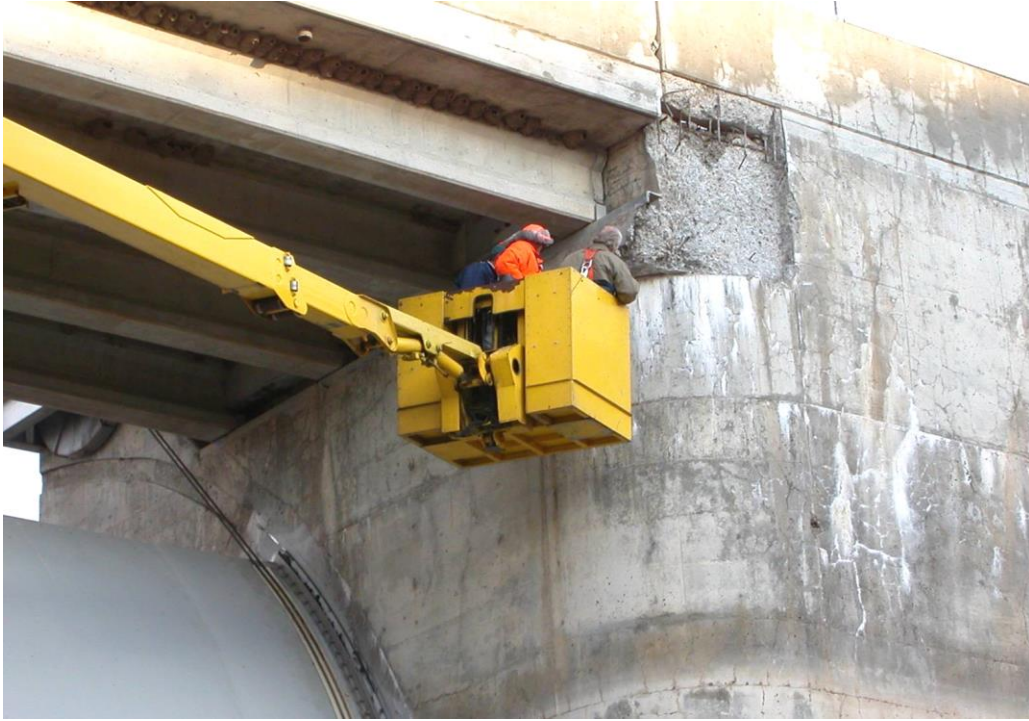
Figure 48. Examining concrete deterioration in a structure built in the 1970s. It was later determined that the deterioration was caused by ASR.
