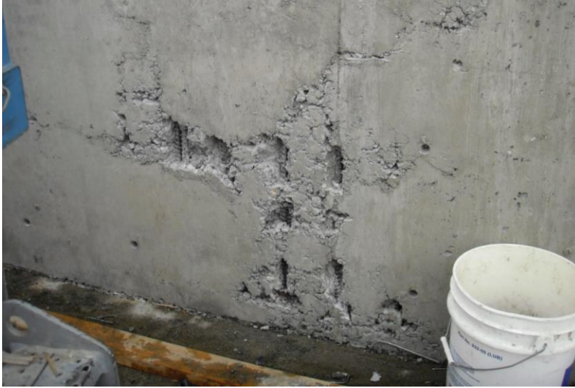
Figure 40. An example of inadequately consolidated concrete that needs repair.
