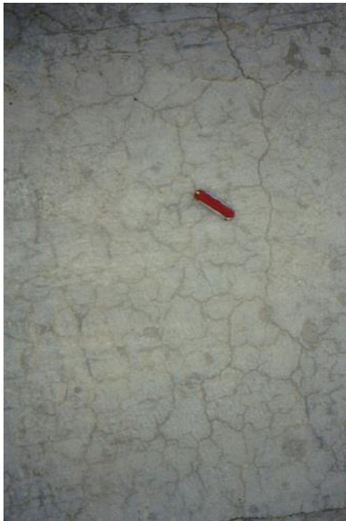
Figure 66. Excessive drying shrinkage cracking due to loss of water from the concrete after hardening.
