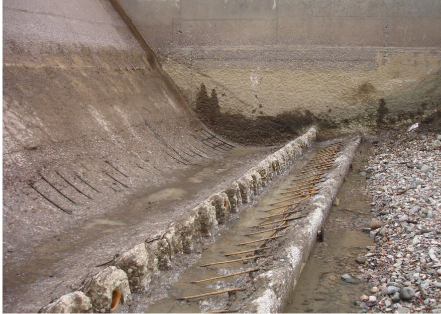
Figure 15. Abrasion erosion damage to the flip bucket and energy dissipaters. The underlying cause of the damage was not determined prior to starting repairs.
