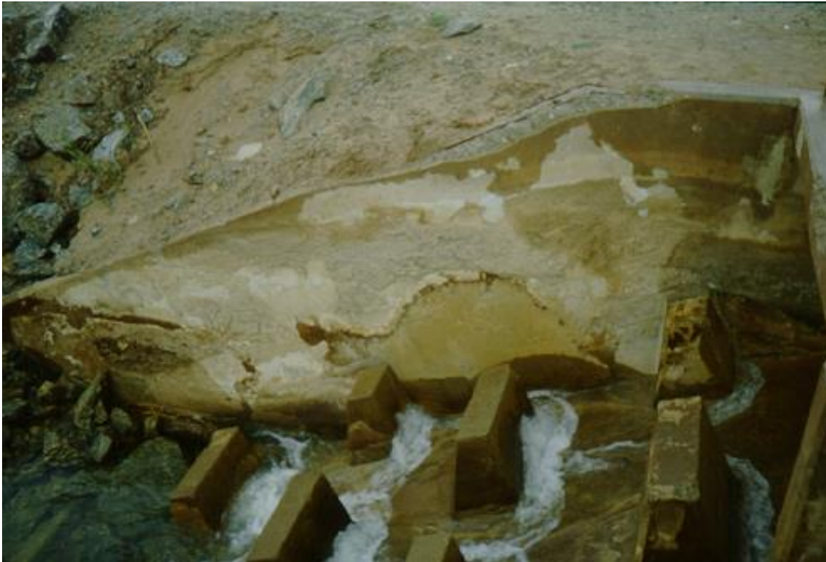
Figure 62. High chlorides in water, leading to corrosion of reinforcing steel.
