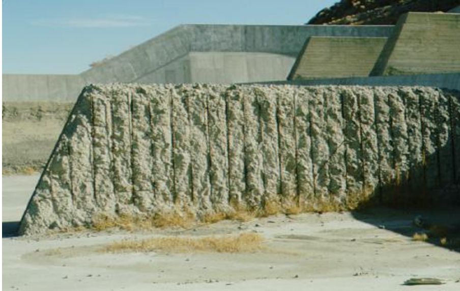
Figure 10. Freeze-thaw damage that should have been repaired before damage became so extensive.
