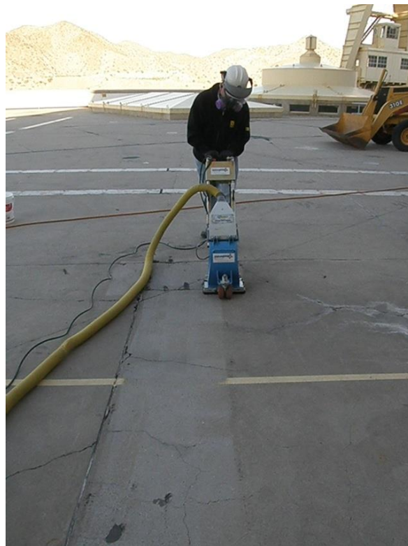
Figure 25. Shotblasting using a small unit prior to application of a healer-sealer (Sealers and Coatings). Even though this unit is small, it is capable of preparing a large area fairly quickly.
