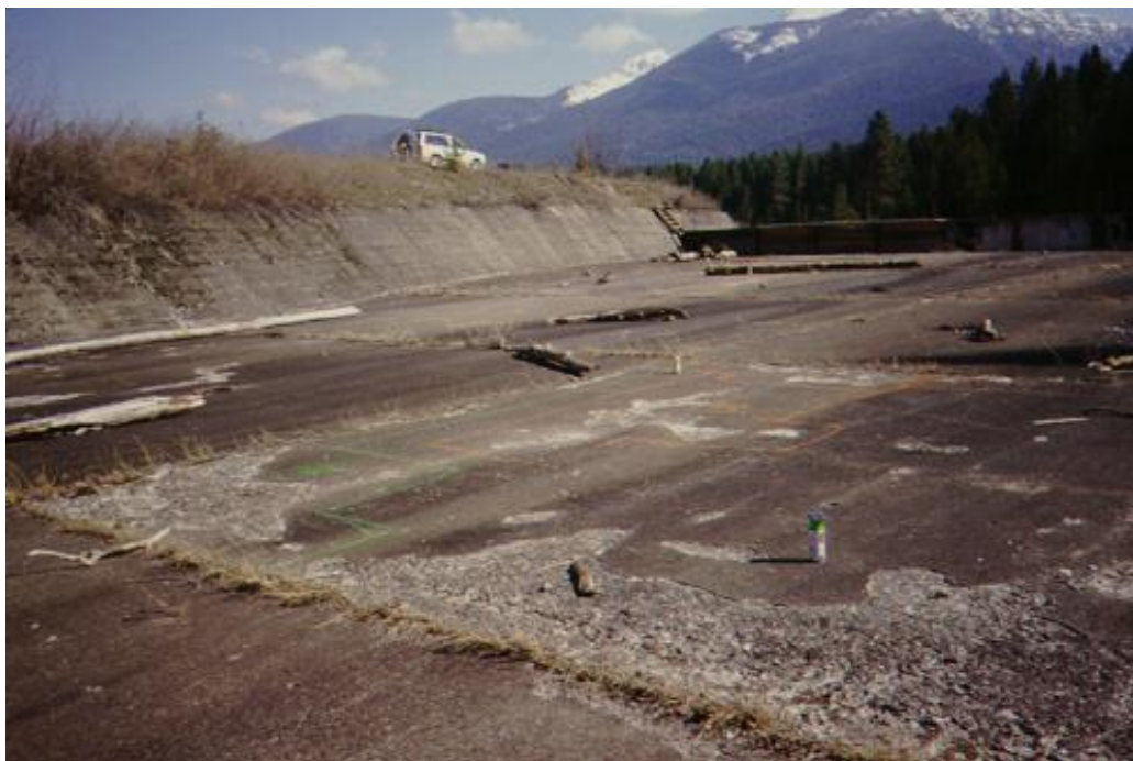
Figure 51. Another example of freeze-thaw deterioration. It is common for the damage to be more pronounced at joints because they will likely stay saturated longer.
