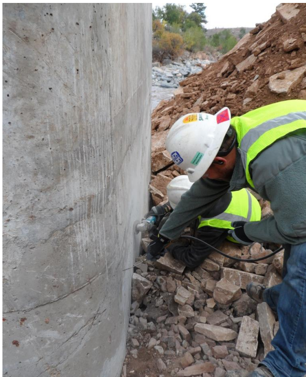
Figure 112. Using compressed air to clean dust and debris from the crack opening.
