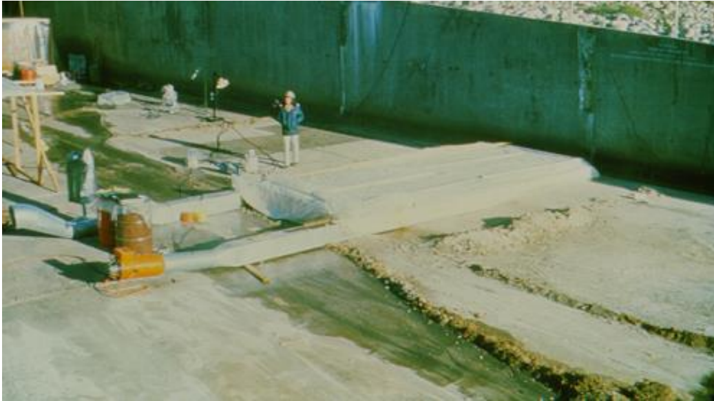
Figure 97. Applying heat to speed curing of a polymer concrete repair. Note the soil berms to prevent water from flowing into the repair area.
