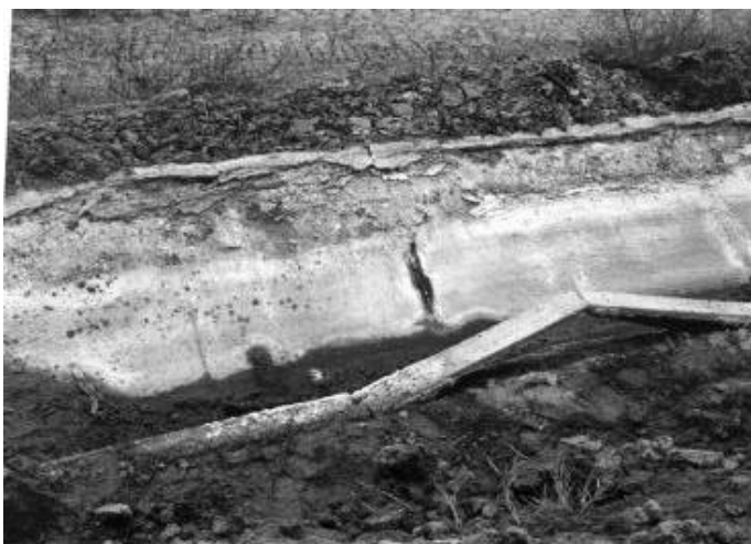
Figure 1. Sulfate attack on a 5-year-old concrete canal lining, Central Valley Project, California. The ground water sulfates infiltrate the concrete and chemically react with certain cement hydration products. The expansive reaction causes cracking.
