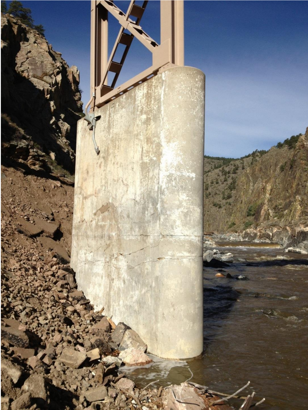
Figure 75. Structural damage from a collapsed roadway that impacted a pier of a siphon. The road was undercut by flooding and then collapsed against the pier. Structural analysis indicated that the reinforcing steel was not yielded, so epoxy injection was used to repair the pier.
