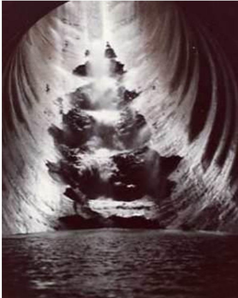
Figure 59. Typical pattern for cavitation damage in a spillway tunnel.
