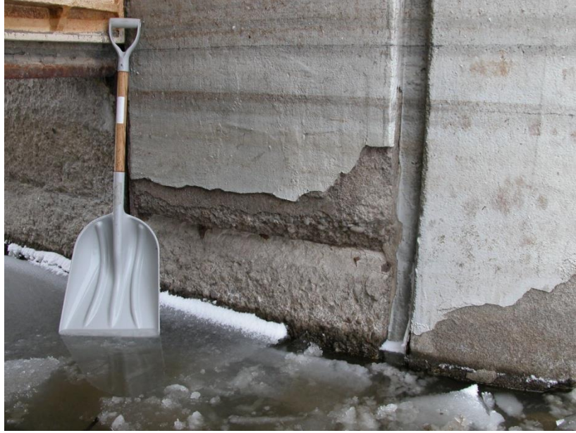
Figure 53. Repairs that were not thick enough to prevent cycles of freezing and thawing weather from damaging the underlying concrete.
