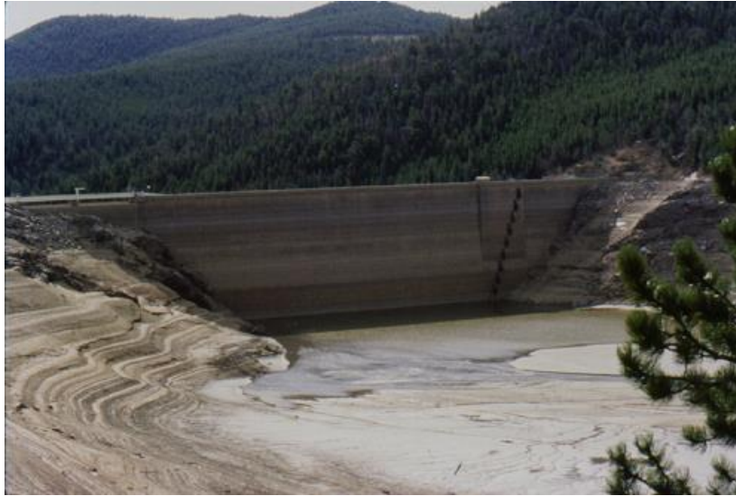
Figure 103. The upstream face of Barker Dam was repaired with a combination of precast panels and preplaced aggregate concrete.
