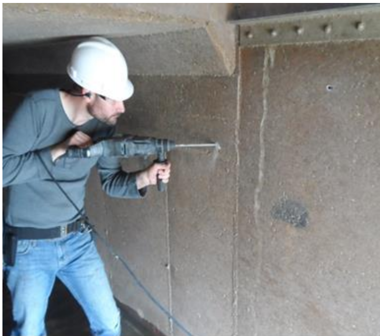
Figure 115. Drilling an injection hole to intercept the leak several inches from the face for polyurethane resin injection.
