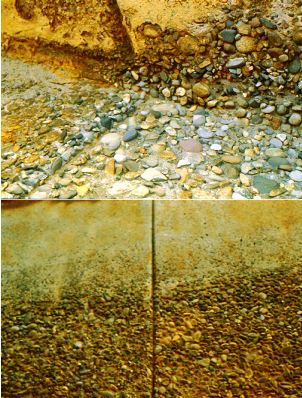
Figure 63. Examples of acid exposure on concrete.
