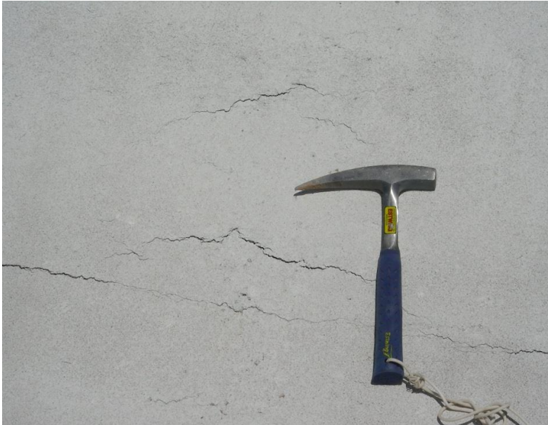
Figure 67. Plastic shrinkage cracking in concrete placed in hot, dry weather.
