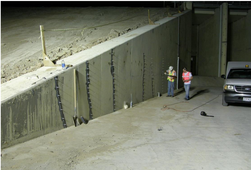
Figure 35. Thermal cracking in a thick concrete wall. The concrete got fairly hot during curing and then cooled too quickly. The picture shows epoxy resin injection repairs underway.
