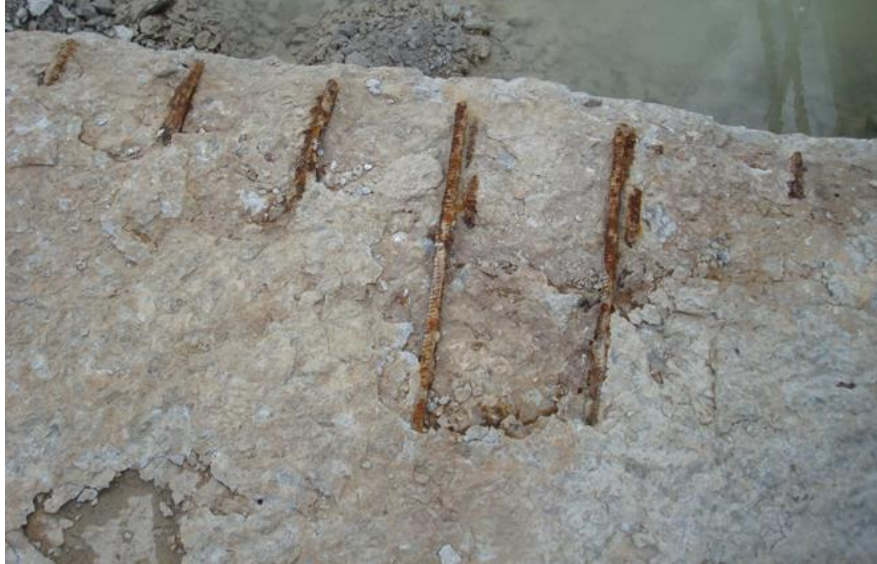
Figure 5. Poor quality aggregate used in concrete placed in the late 1960s led to the need for expensive repairs in the 2000s.
