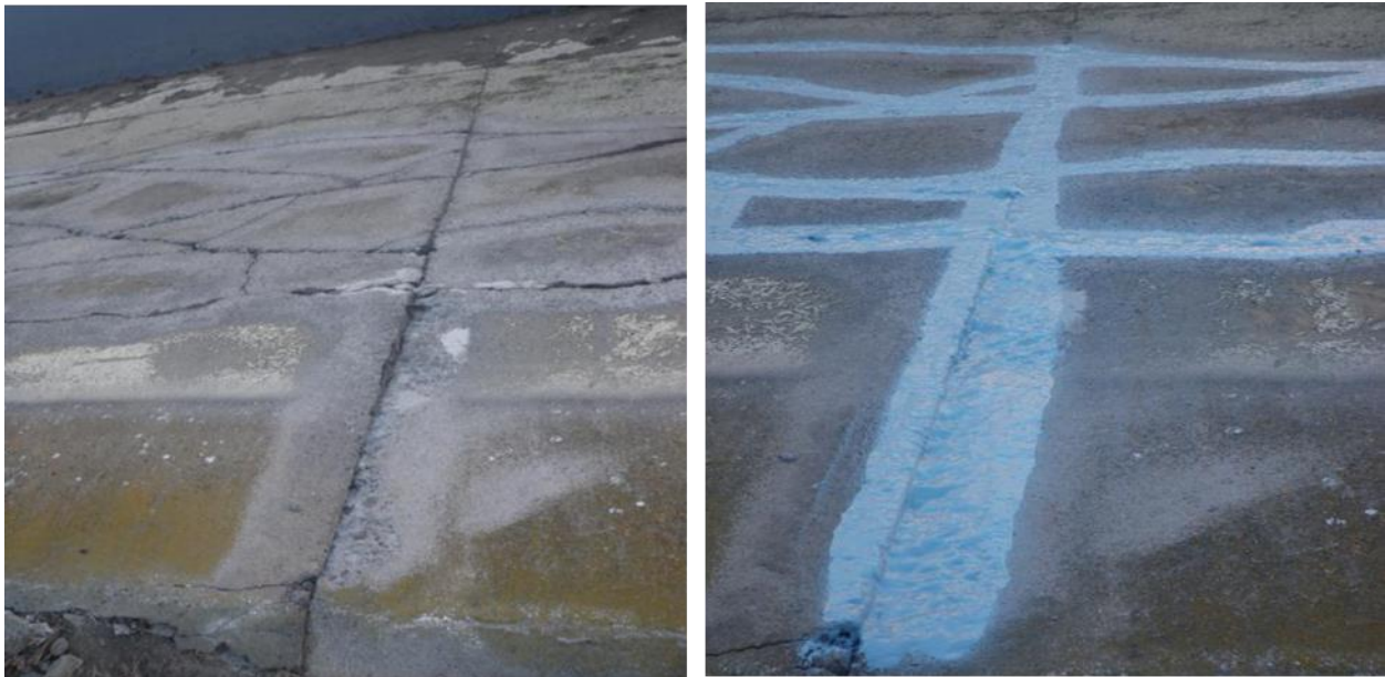
Figure 83. Cracked concrete canal lining repaired with an elastomeric polyurea.
