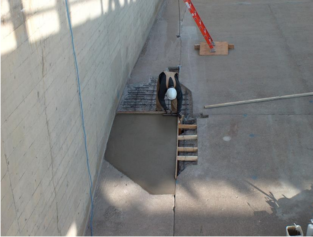
Figure 4. Formwork used to maintain the existing joints in a spillway floor repair.
