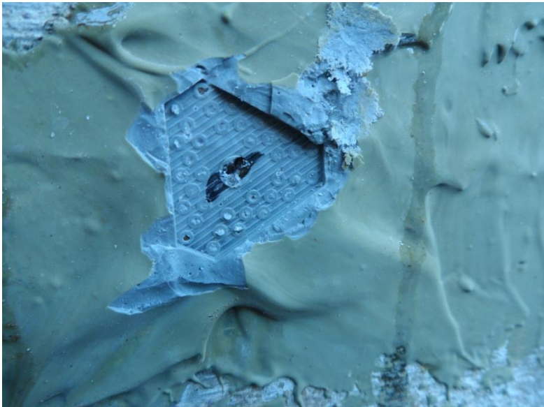
Figure 125. The exposed crack, after removing the injection port, is filled with cured epoxy.
