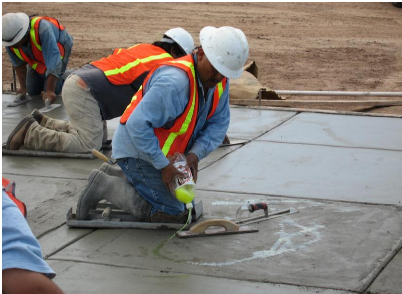
Figure 41. The addition of water or other substances during finishing can lead to weakened and damaged concrete surfaces.
