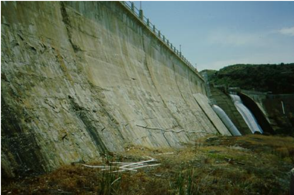
Figure 9. A structure experiencing freeze-thaw deterioration that will not need repair for many years.
