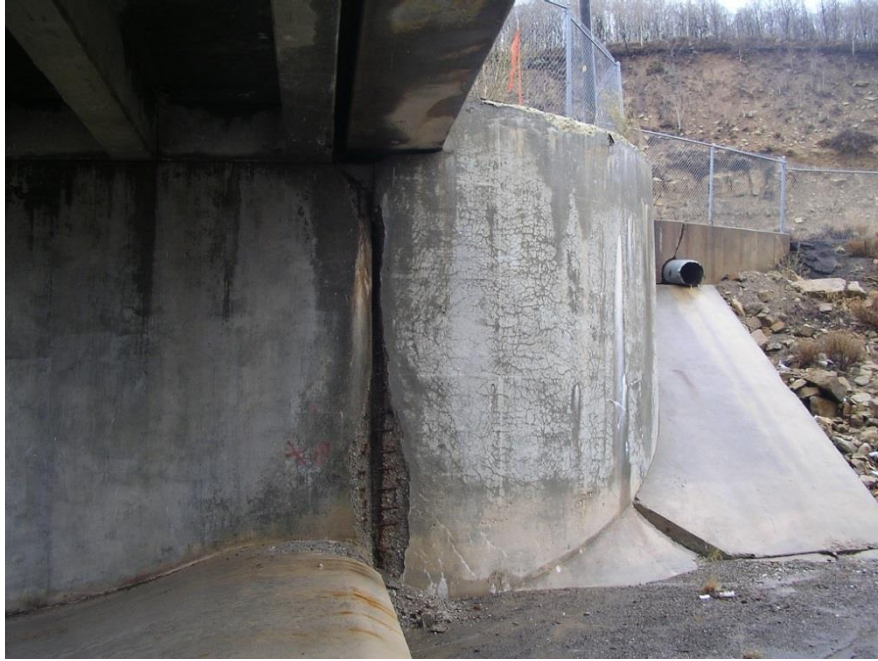
Figure 36. Corrosion of reinforcing steel from deicing salts used on the bridge.
