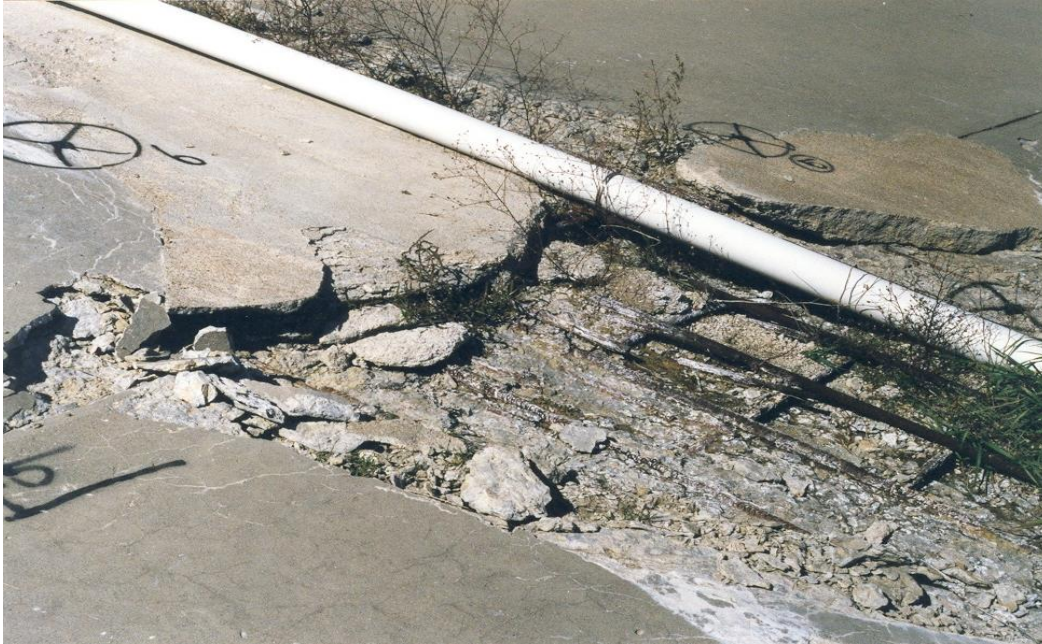
Figure 44. Repairs that were damaged by sulfate attack. New repairs were performed using materials that are durable when exposed to sulfates.
