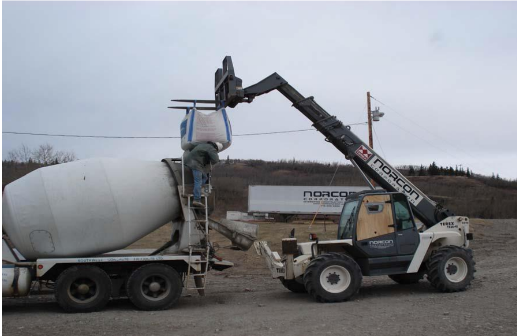
Figure 58. High-strength silica fume concrete materials were delivered in 3,000-pound sacks and mixed onsite with water and liquid admixtures.
