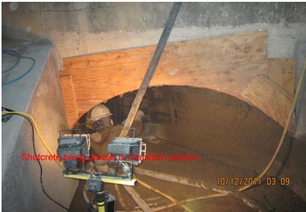
Figure 105. Even though space was limited, due to the complicated geometry of this outlet works, shotcrete was used to make concrete repairs. The shotcrete was later finished to a smooth surface.
