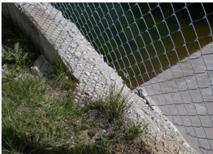
Figure 50. The top of a spillway wall suffering damage from cycles of freezing and thawing weather.
