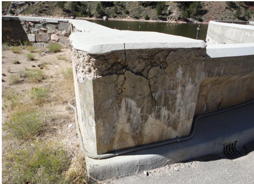
Figure 47. Extensive cracking which can indicate ASR.
