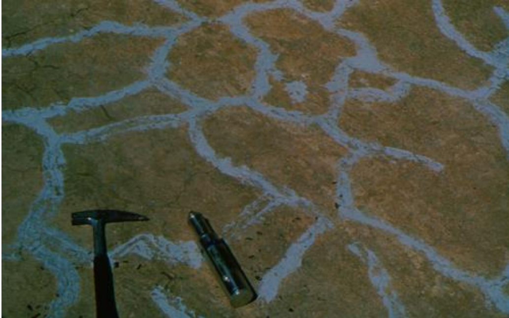
Figure 71. An example of improper crack repair, resulting in an unsightly appearance.
