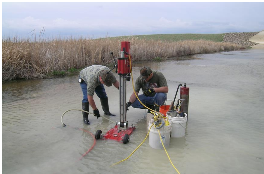
Figure 6. Obtaining concrete samples is very important to properly assess the cause and extent of damage. In this case, the concrete apron was a few inches below the water surface.
