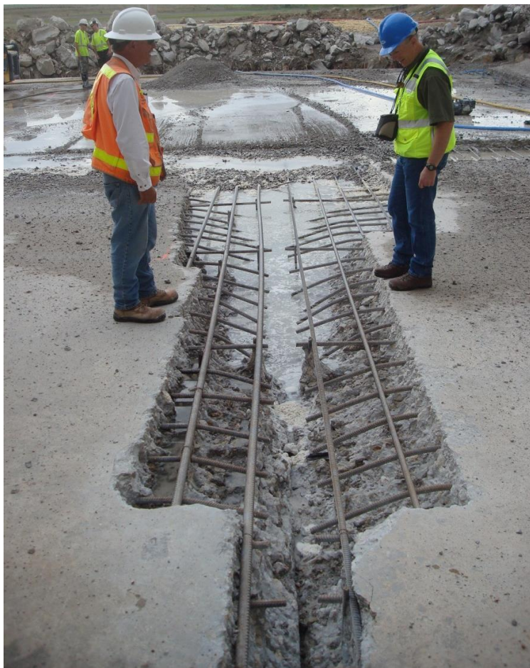
Figure 23. The first calibration test resulted in excessive concrete removal and bent rebar.
