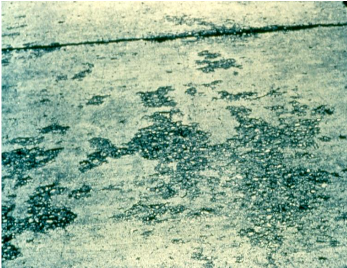
Figure 42. Surface damage appearing in new concrete caused by the addition of water during finishing.
