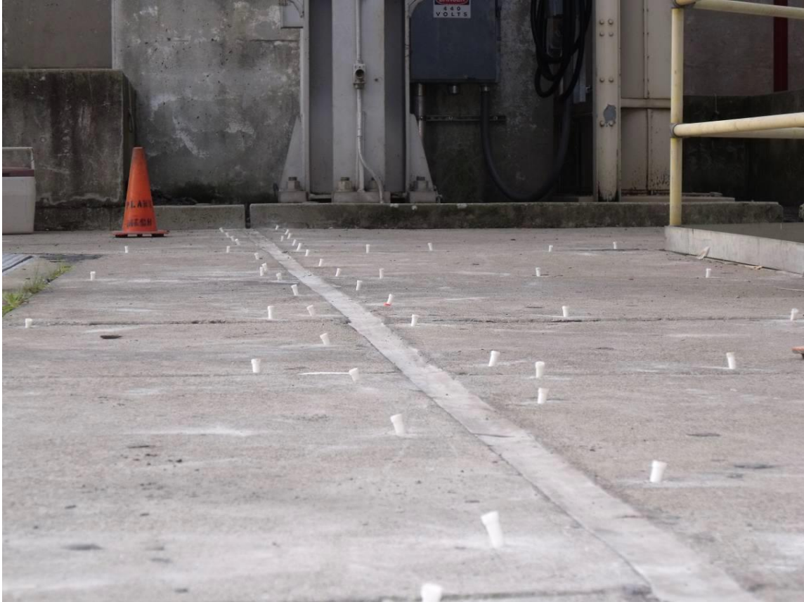
Figure 116. Ports placed into holes for injecting polyurethane resin into a leaking expansion joint in a powerplant deck. The holes are drilled to intercept the joint between the rubber waterstop and an embedded metal plate.
