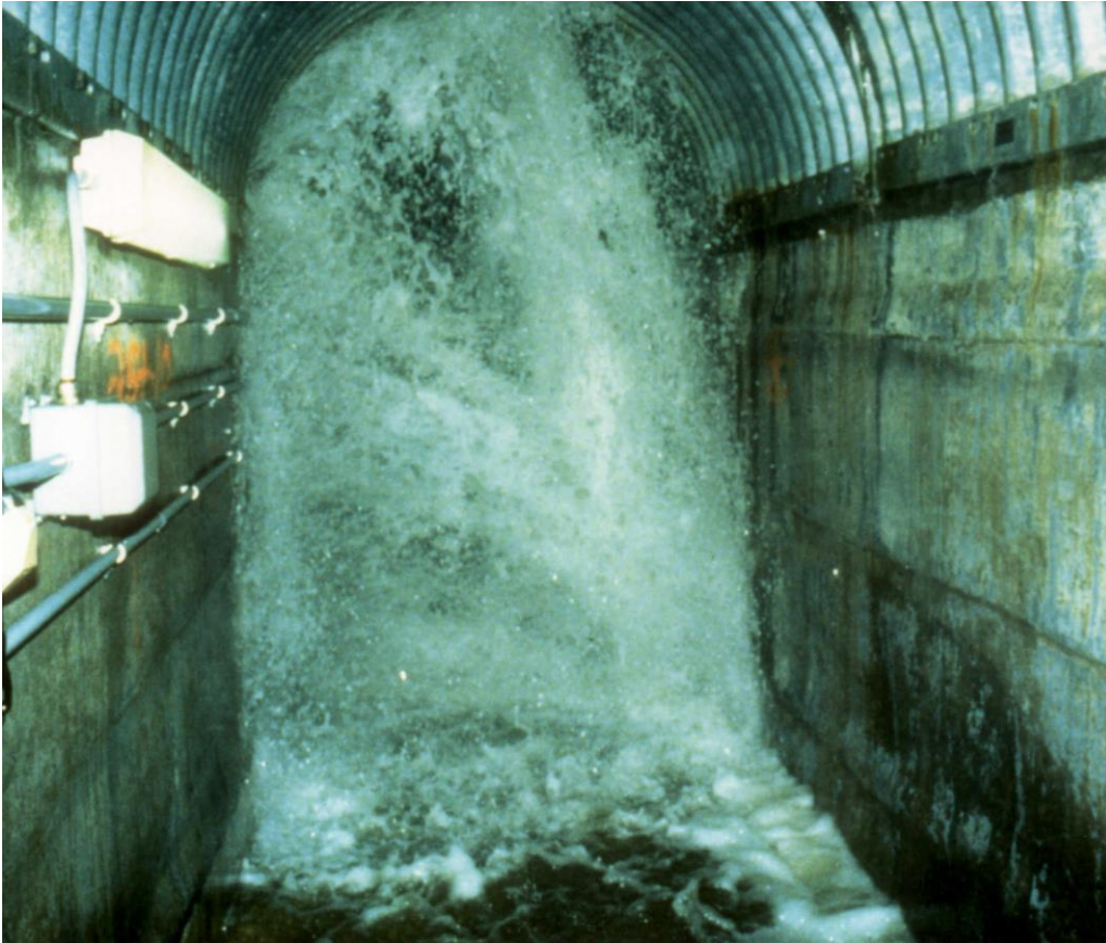
Figure 109. High-volume water leaks can be repaired using polyurethane resins.
