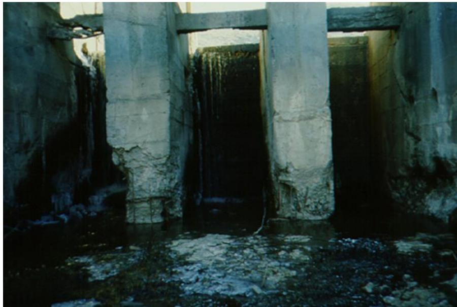
Figure 1. Freeze-thaw damage that could have been prevented by proper maintenance.
