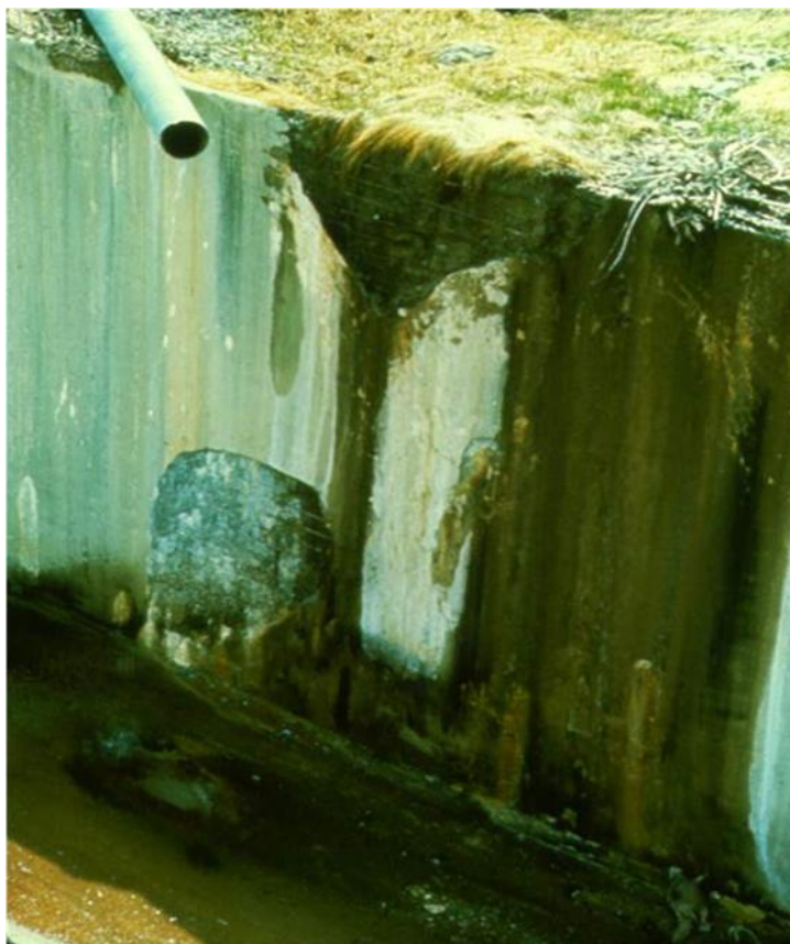
Figure 2. Removing the source of water properly would have resulted in significantly less damage.
