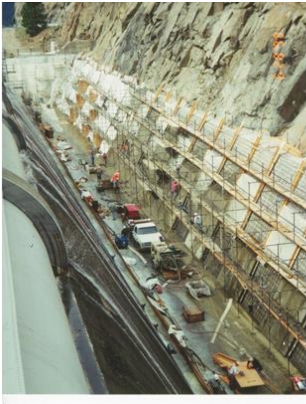
Figure 8. Tieton Dam spillway reconstruction in 1999, Yakima Project, Washington. The challenge for the 21st century: identify, protect, and preserve. The spillway was completed in 1925 and suffered from severe FT deterioration. It was extensively repaired after about 40 years and reconstructed in 1999. These types of rehabilitation efforts will take center stage in 21 st -century Reclamation construction. (Construction records, Yakima Construction Office, Washington)
