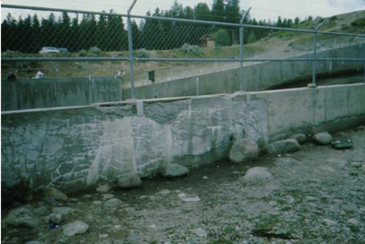
Figure 52. Example of D-cracking that resulted from freezing and thawing weather damage to absorptive aggregates.
