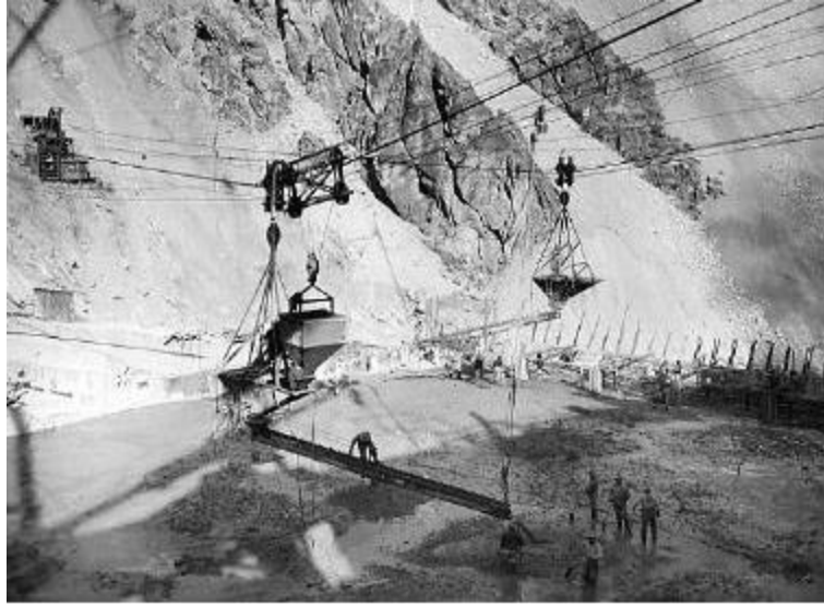
Figure 4. Chuting wet concrete into place at Arrowrock Dam (about 1912). Elaborate chute systems required a very fluid concrete mixture to be placed and spread in the forms. Water was the “admixture” of choice to improve the fluidity! (Bureau of Reclamation historical photographs)
