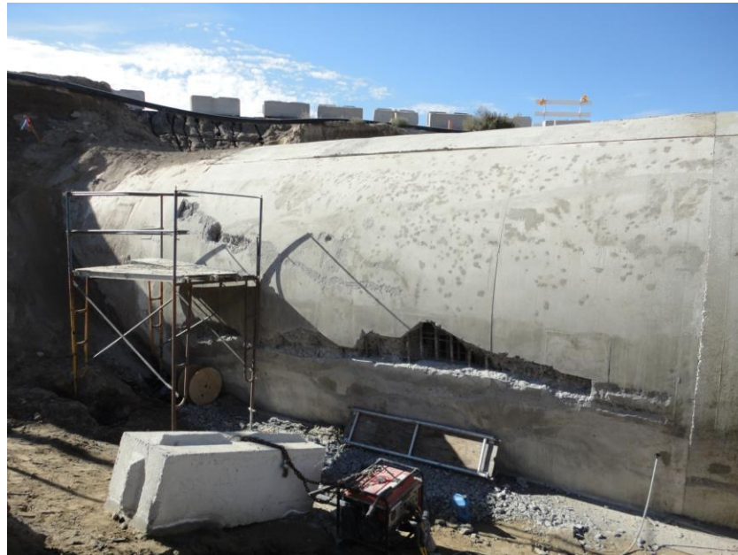
Figure 39. Large voids, rock pockets, and honeycombs resulting from inadequate concrete consolidation.
