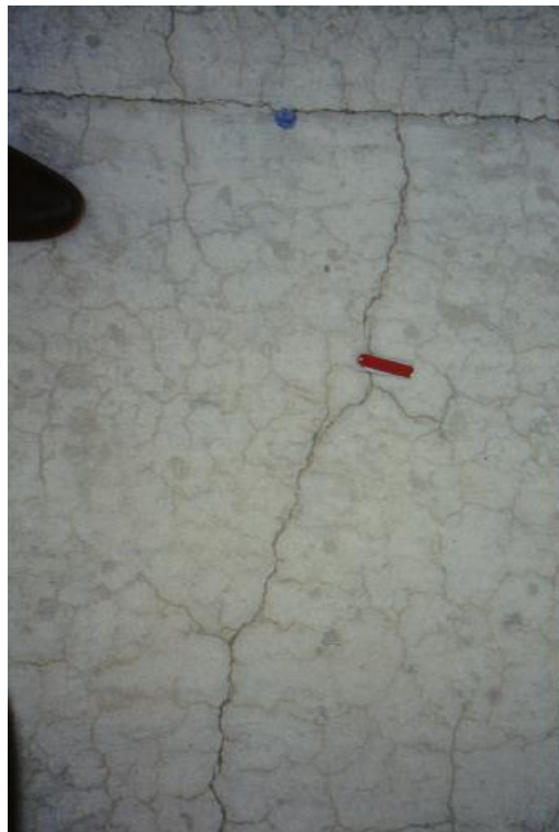
Figure 73. Reflective cracking from cracks below the concrete overlay.
