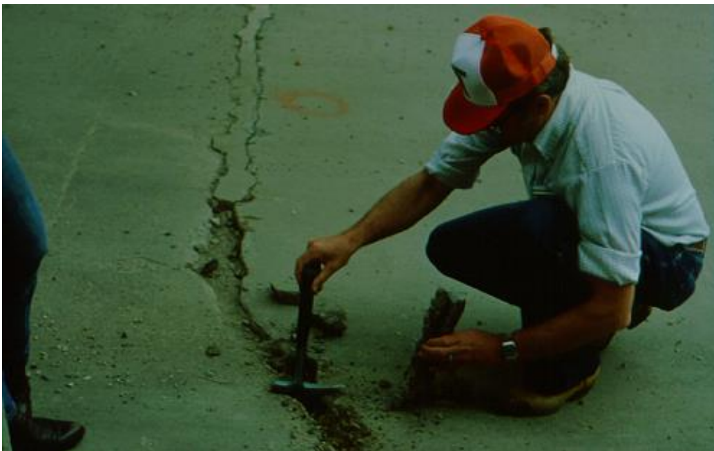
Figure 72. Improperly repairing cracks often makes the repair very short lived.
