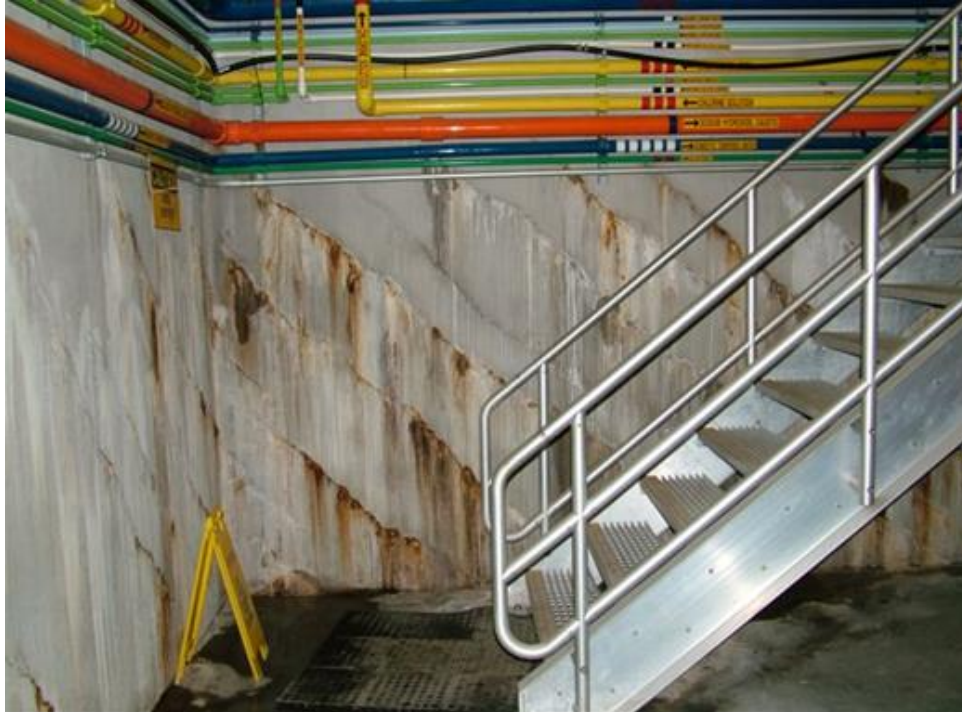
Figure 68. Foundation settlement in this water treatment plant caused cracking in one of the water bays.
