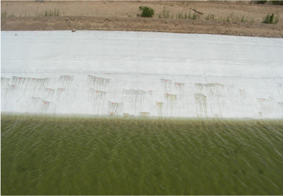
Figure 78. A low viscosity epoxy resin was poured into plastic shrinkage cracks. Although unsightly, the resin was effective in filling and sealing the cracks.
