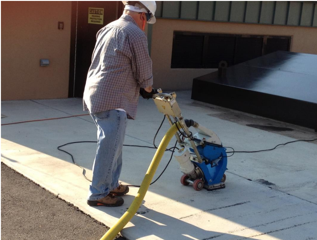
Figure 81. Steel shotblasting a concrete deck prior to application of an epoxy sealer.
