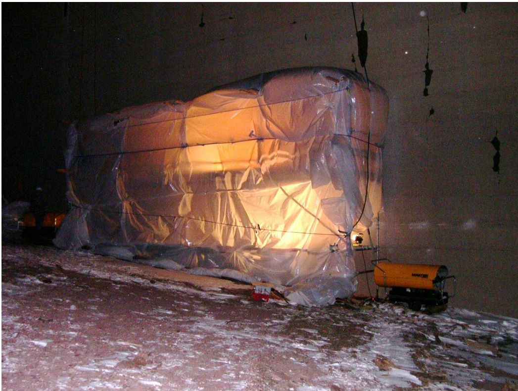
Figure 90. Using heaters in an enclosed area to increase the temperature to meet application requirements.
