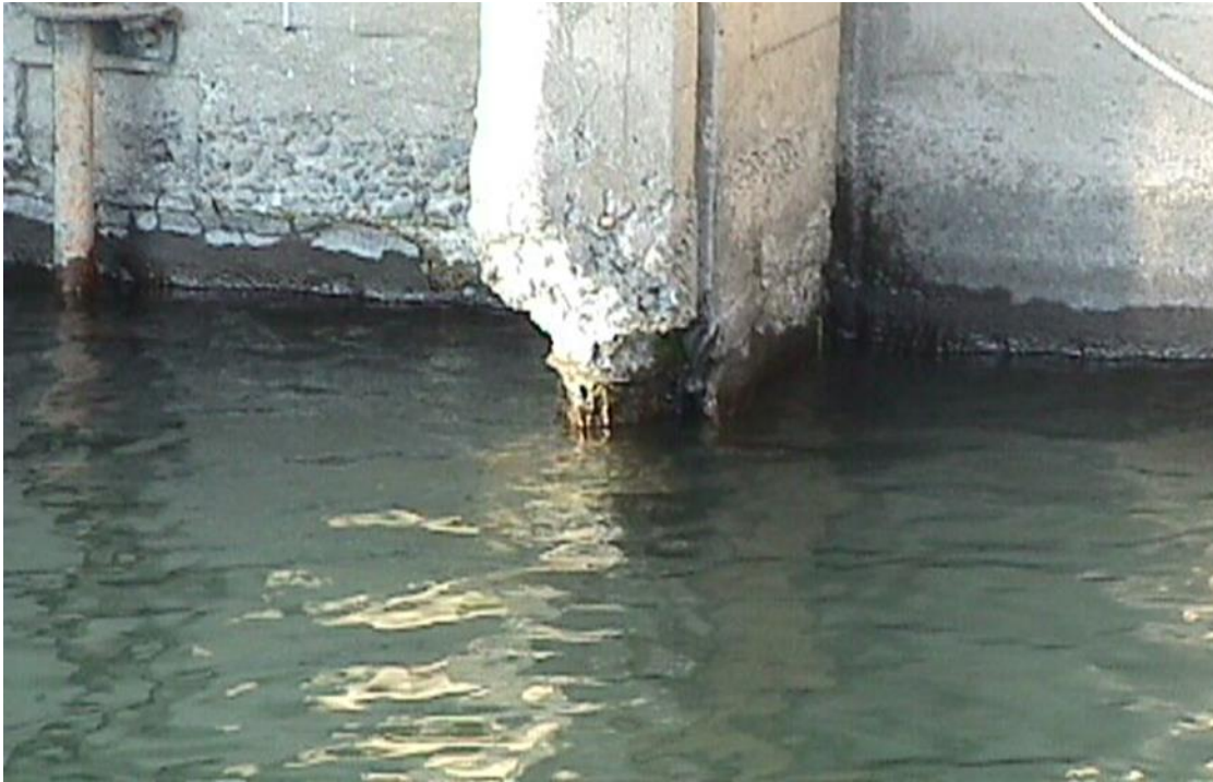
Figure 3. Freeze-thaw damage that could have been reduced by changing operation of the structure.
