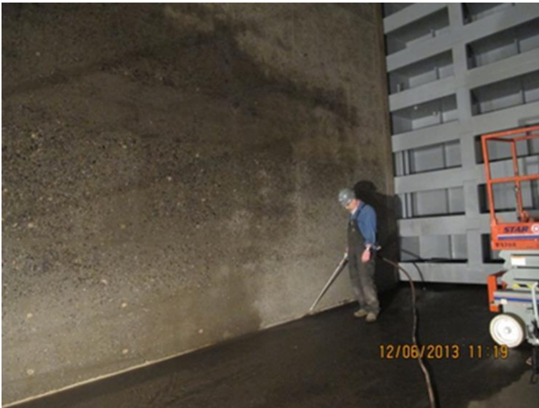
Figure 89. Drying the surface of concrete using oil-free compressed air to meet the surface moisture requirements of the manufacturer.
