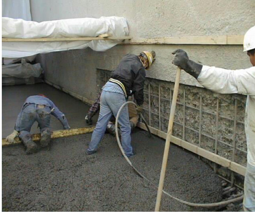
Figure 57. Placing silica fume concrete in a stilling basin in central Colorado to repair abrasion-erosion damage.
