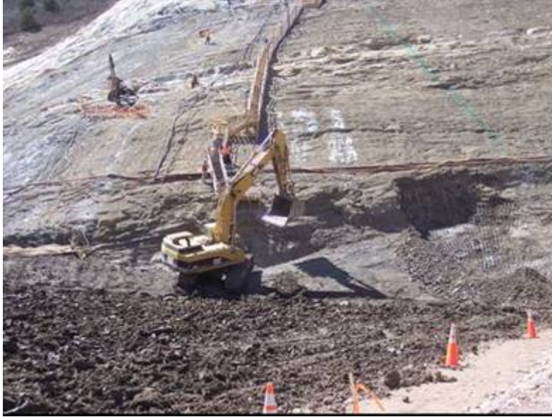
Photograph 4. Caterpillar 365 excavator beginning the additional excavation on the right abutment to remove fractured Lewis Shale. May 1, 2006 (Photo by J. Gates)
