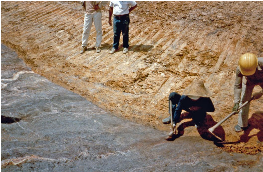
Figure 3.4.2-7 Feather edge of first lift of compacted fill removed, cleaned, and ready for fill placement.
