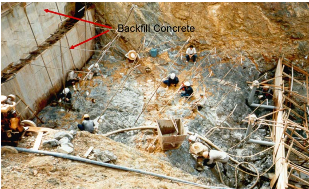
Figure 3.2.6.1-1. Foundation cleanup is labor intensive and costly but should not be neglected.
