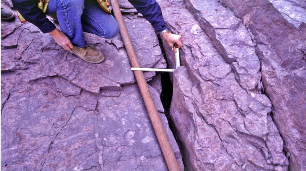
Figure 3.2.4.2-10 Ridges Basin Dam. Open stress relief joint in foundation requires filling with slush grout.
