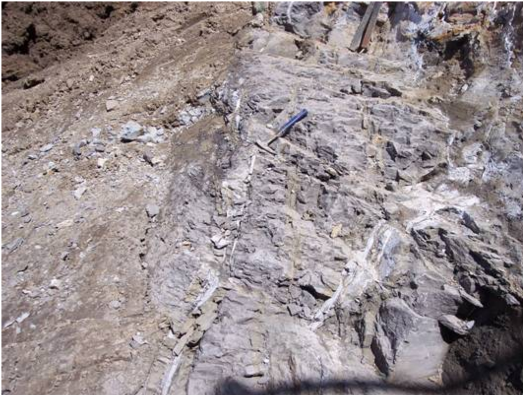
Photograph 6. Joint on right abutment near Station 14+55, 130' US that is filled with grout from foundation pressure grouting operations. The grout reaches a maximum thickness of about 3/4 inch. Grout can also be seen along a joint at the upper right of photo. View looking downstream. April 27, 2006 (Photo by R. Christianson) Reference Image Only
