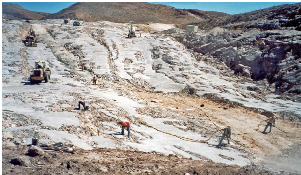
Figure 3.2.4.2-3 Extensive use of dental concrete used to fill potholes, grooves, and channels in rock surface.
