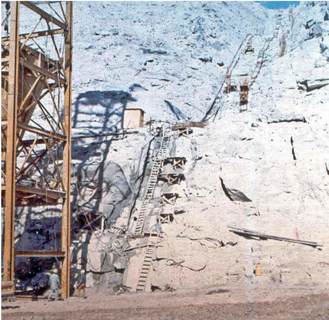
Figure 3.2.4.2-9 Teton Dam. The stepped surface in this right abutment key trench could result in cracking and seepage problems in overlying embankment. Embankment may differentially settle adjacent to these surfaces, resulting in cracks.
