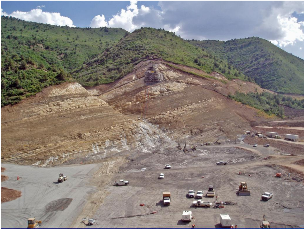
Figure 3.2.4.2-2 Ridges Basin Dam. This dam foundation was shaped to ensure proper compaction of fill and to prevent stress irregularities in the overlying embankment.
