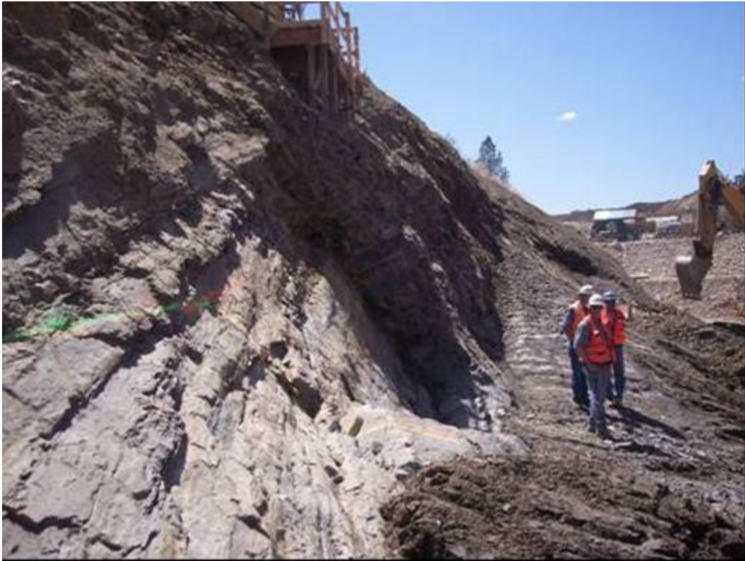
Photograph 3. Upstream view of fractured rock prior to additional excavation taking place above approximate elevation 6665 on the upstream right abutment. Geologist and inspectors are standing at approximate Station 14+55, 135' upstream of centerline. April 27, 2006 (Photo R. Christianson)
