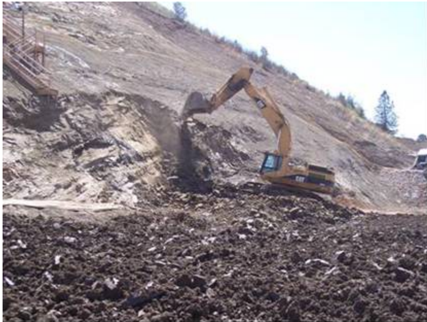
Photograph 5. Additional excavation is being accomplished using a Caterpillar 365 trackhoe and is exposing a prominent joint face on the upstream right abutment. The excavator can be seen working on the upstream transition. May 10, 2006 (Photo by J. Gates)
