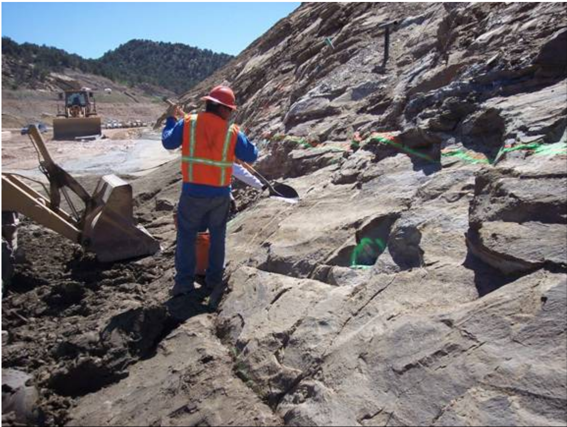
Photograph 7. Slush grout being placed in preparation for Zone 1 embankment. This area represents the gradational contact between the Lewis Shale and the overlying Pictured Cliffs Unit P1. View looking downstream from approximate Station 15+00 40' U/S. May 24, 2006 (Photo by R. Christianson) Reference Image Only
