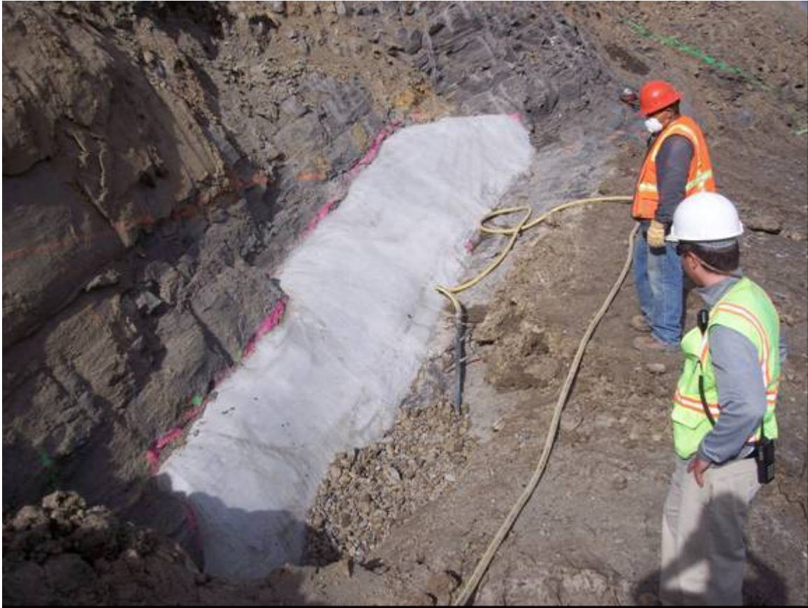
Photograph 6. Unformed dental concrete at the base of the exposed joint face on the right abutment between approximate Stations 14+15, 168' US and 14+98, 190' US. May 22, 2006 (Photo by J. Gates)
