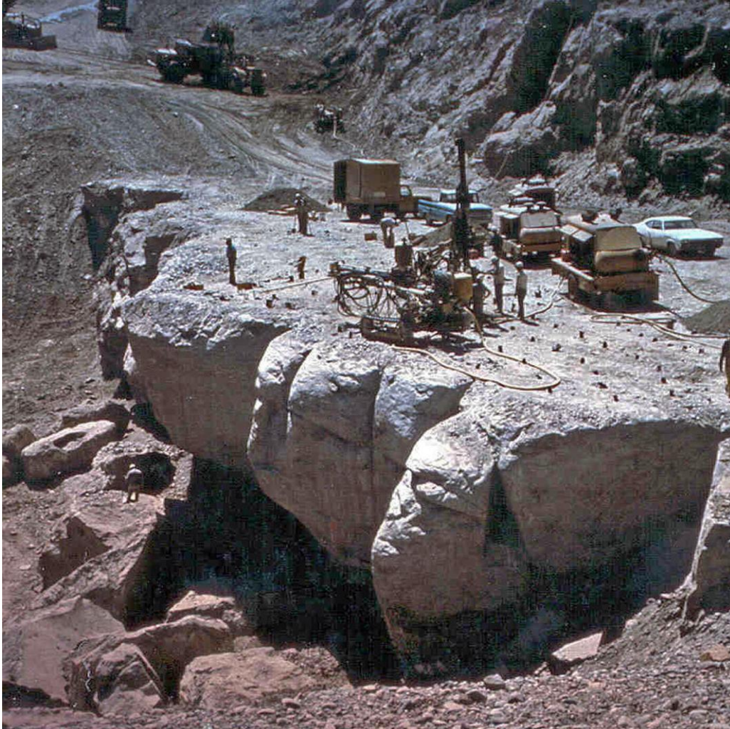
Figure 3.2.4.2-8 Drilling blast holes to facilitate removal of a rock overhang at Teton Dam.
