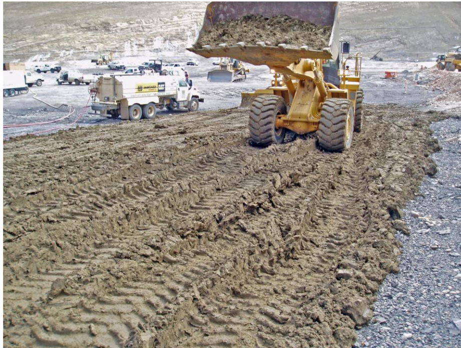
Figure 3.4.2-2 Pneumatic-tire equipment should be used to compact fill near the foundation contact surfaces. A sheep's foot or tamping roller may be used when the fill is thick enough to prevent contact of the tamping feet with the foundation.
