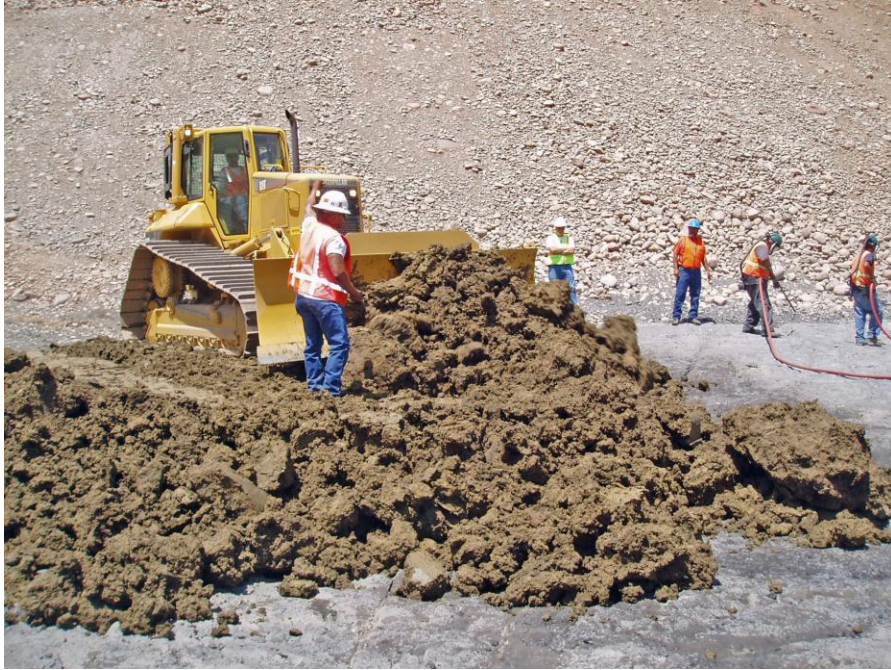
Figure 3.4.2-6 Ridges Basin Dam. Final foundation cleanup and spreading first lift. Note the dozer is working on the fill, not on the foundation surface, to prevent foundation damage. Foundation rock in foreground has been moistened.
