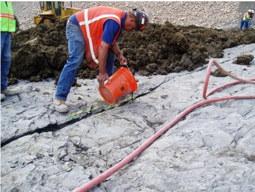
Figure 3.2.4.2-11 Slush grout being applied to an open joint in a dam foundation.
