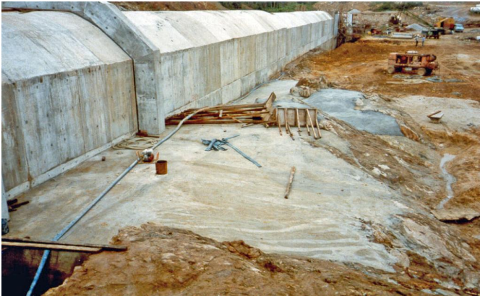
Figure 3.2.6.6-3 Foundation for outlet works structure was shaped and treated with dental concrete.
