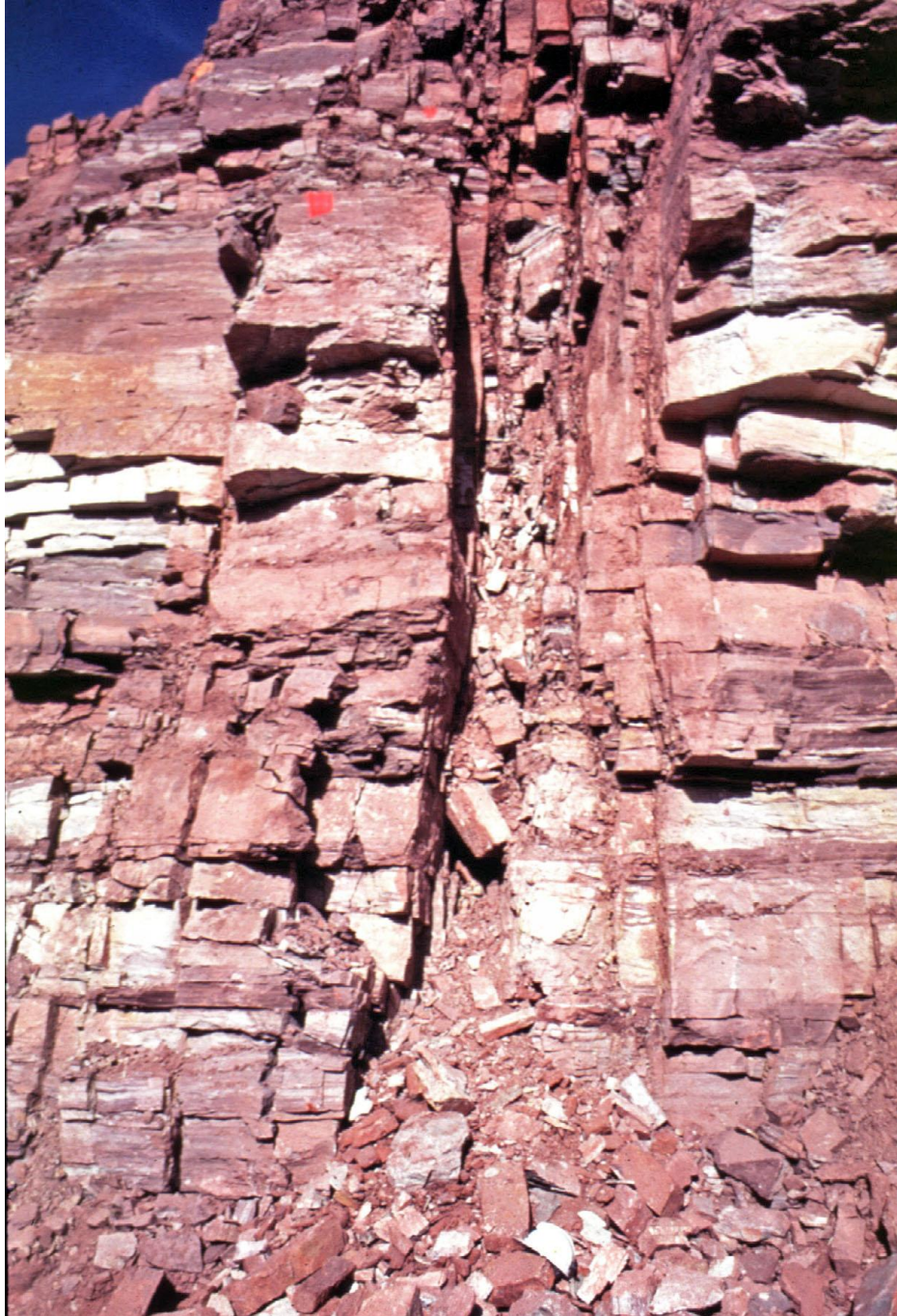
Figure 3.2.4.2-1 Upper Stillwater Dam. Features such as this shear zone create foundation irregularities that require treatment. The surface should be cleaned of all loose and weathered rock, and the shear zone should be filled with dental concrete. Alternatively, the surface might be reformed by smooth blasting techniques.
