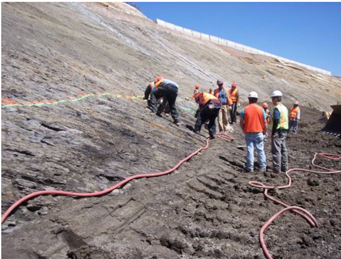
Photograph 2. Crew finishes preparing the foundation for Zone 1 placement on the lower left abutment at approximate Station 22+30, 150' US. View looking downstream. May 5, 2006 (photo by R. Christianson)
