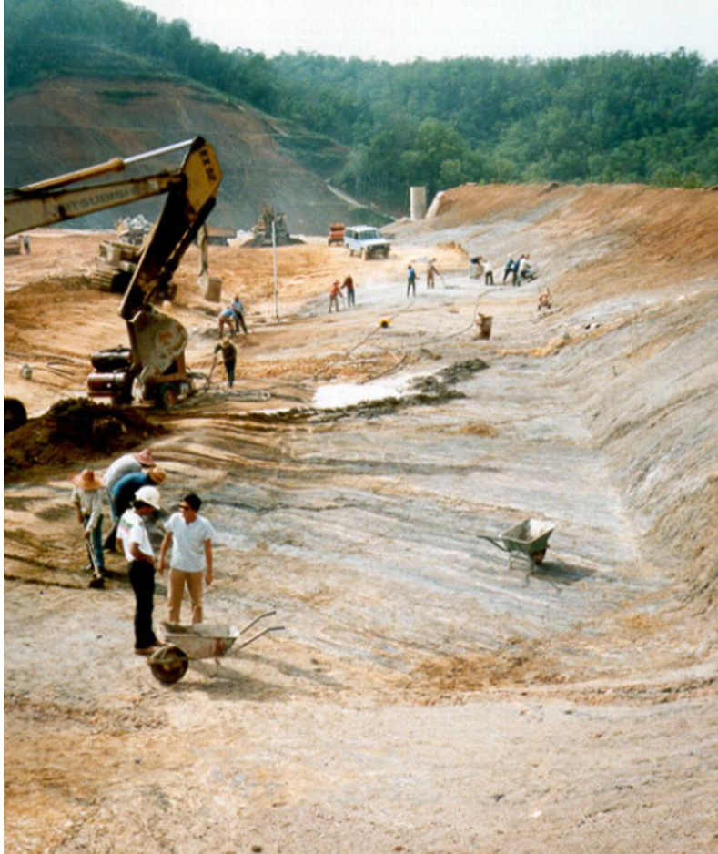
Figure 3.2.1-1 All organic or other unsuitable materials should be removed from soil foundations.
