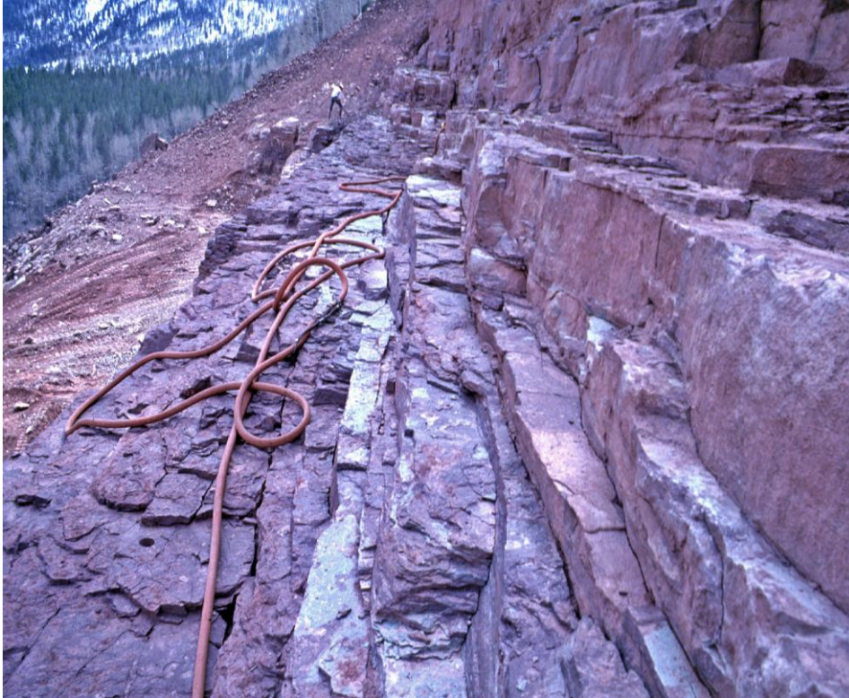
Figure 3.2.6.6-1 Upper Stillwater Dam. Foundation excavated to material capable of withstanding loads imposed by the dam. Left side of photograph shows acceptable steps; right side shows steps requiring concrete fillets.
