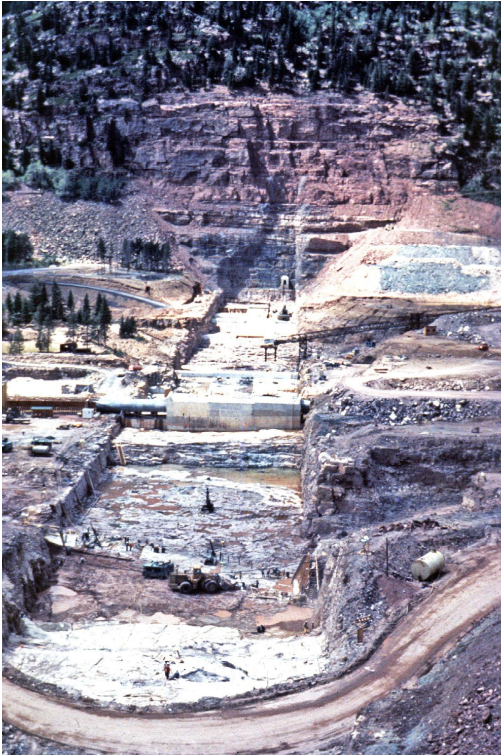
Figure 3.2.6.6-5 Entire footprint of a concrete gravity dam is excavated to material capable of withstanding loads imposed by the dam.
