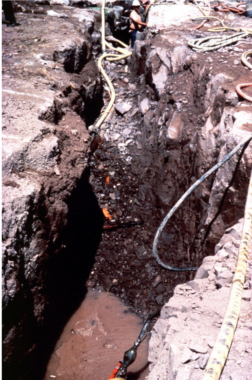
Figure 3.2.4.2-12. Upper Stillwater Dam. Shear zone in foundation being cleaned out for concrete backfill.
