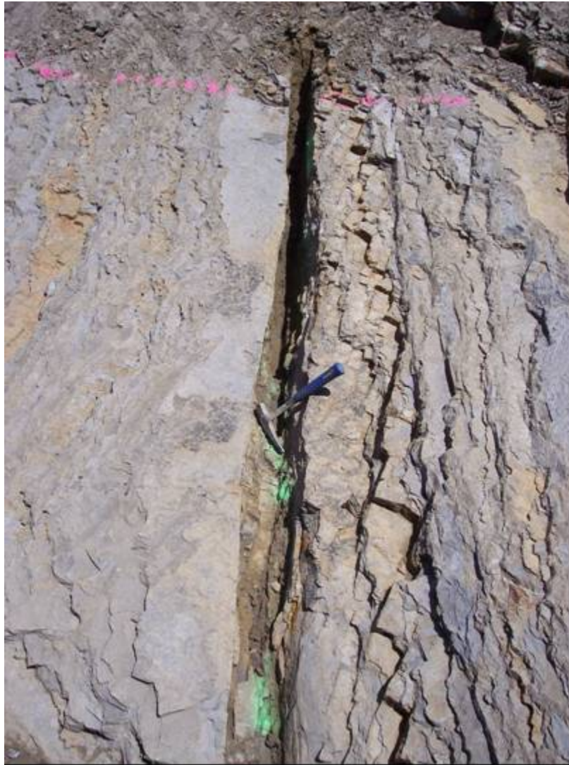
Photograph 1. Weathered rock materials have been excavated from an "A" joint on the left abutment at approximate Station 22+58, 132' US in preparation for slush grouting. The weathered materials have become firm throughout most of the exposed joint at the excavated depth. May 23, 2006 (Photo by J. Gates) Reference Image Only
