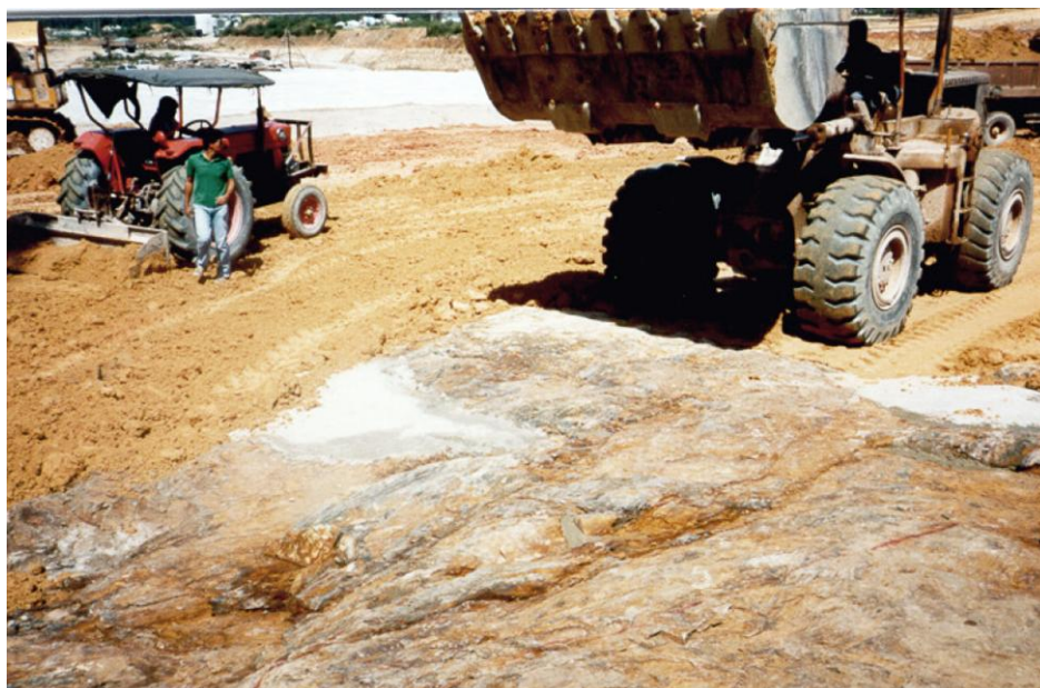
Figure 3.4.2-3 Pneumatic-tire equipment forces the plastic and deformable earthfill into all remaining uneven surfaces in the foundation surface and may create a feather edge at the ends of the placement.
