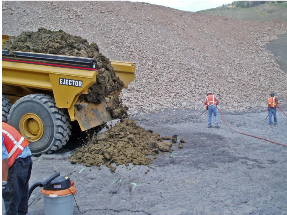
Figure 3.4.2-4 Ridges Basin Dam. Final foundation cleanup and placing the first lift of embankment fill.
