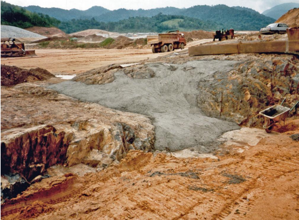
Figure 3.2.6.3-1 Dental concrete and acceptable vertical steps can be tolerated in the foundation.
