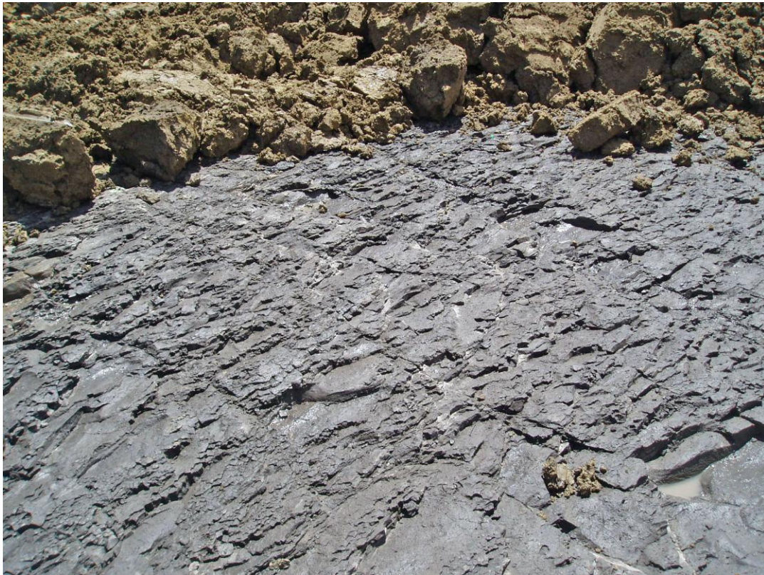
Figure 3.4.2-1 After final cleanup, the foundation is moistened prior to placing and compacting embankment fill.
