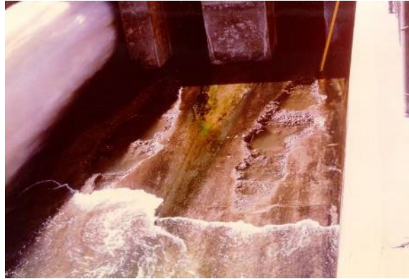
Cavitation damage downstream of regulating gates (Palisades Dam, Wyoming).
