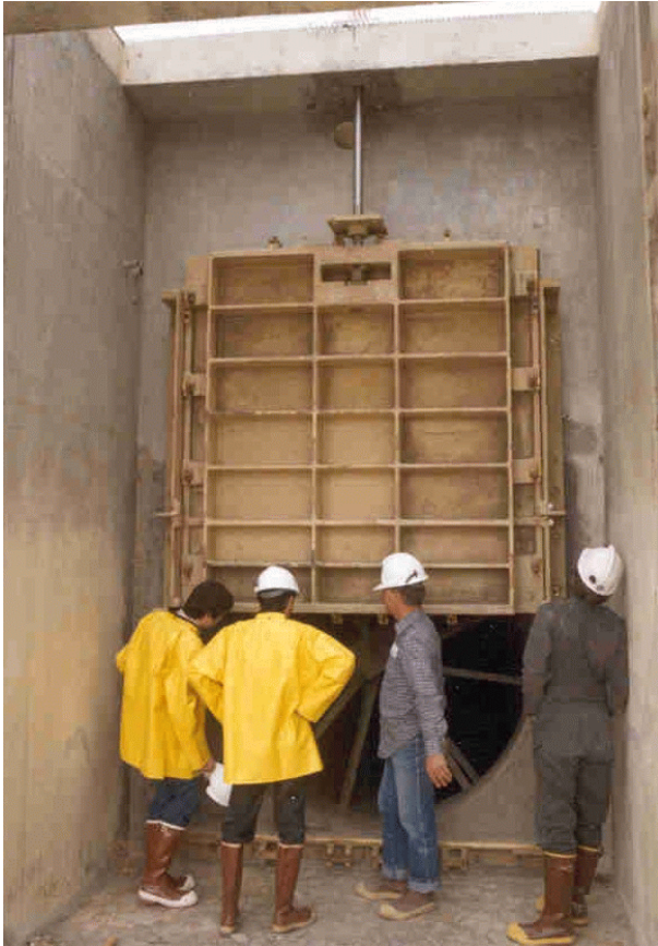
Figure 4.9.1.1-17. Unbonneted slide gate.
