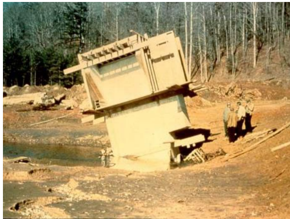
Outlet works intake tower tilting due to inadequate foundation support (unknown dam).
