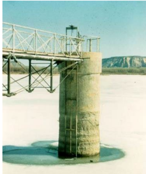
Outlet works intake tower deterioration due to freeze-thaw cycles and ice action (unknown dam).
