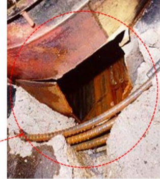
1997 cavitation-induced pipe failure due to ring-follower gate leaf drifting into flow (Flaming Gorge Dam).
