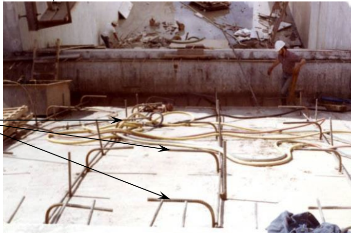
Constructing new outlet works. Note anchor bars installed through mud slab into foundation associated with outlet works chute.
