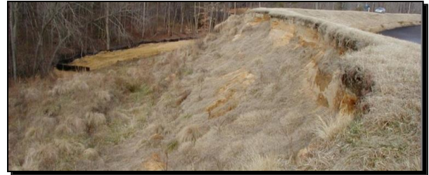
Photo 6: Deep slide, slump, and slips on a slope (ASDSO)
