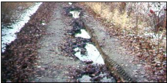
Photo 16: Crest ruts (ASDSO)
