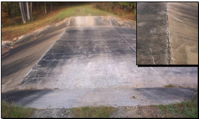
Photo 1: Concrete spillway from the inspection report. Photo inset shows an open joint.
