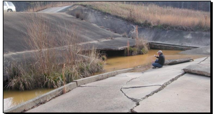
Photo 2: Failed concrete spillway following operation during a storm event.
