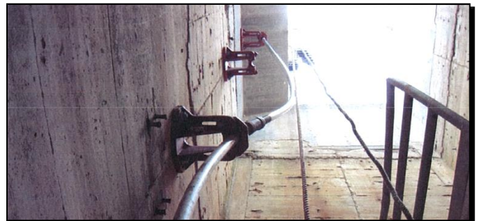
Photo 21: Bent gate stem (AECOM)
