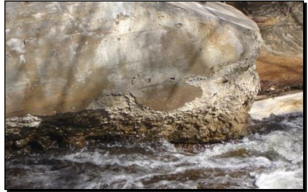
Photo 20: Concrete erosion (AECOM)
