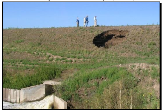
Photo 7: Sinkhole on downstream slope (AECOM)
