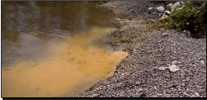
Photo 18: Muddy seepage at downstream toe (ASDSO)
