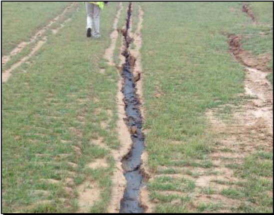
Photo 9: Slope erosion and sparse vegetation (AECOM)
