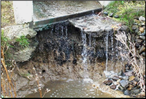
Photo 22: Erosion and undermining of outlet structure (AECOM)
