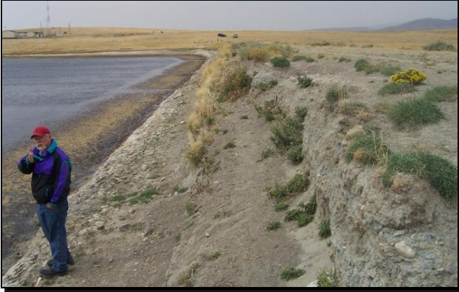
Photo 8: Loss of riprap and slope erosion (Montana DNRC)
