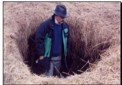
Photo 13: Crest sinkhole (ASDSO)
