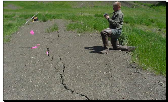
Photo 12: Longitudinal crest crack (Montana DNRC)
