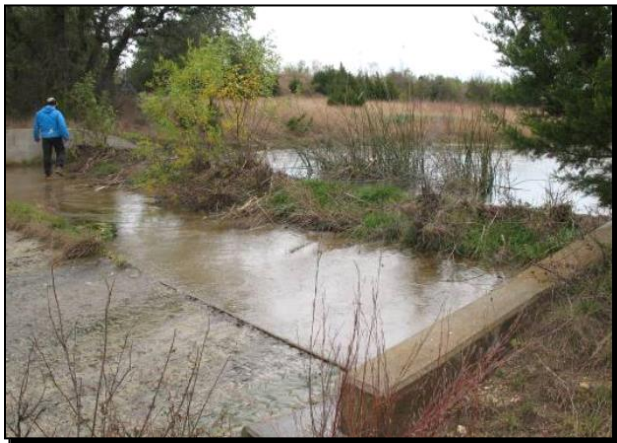
Photo 19: Vegetation obstructing spillway flow (AECOM)
