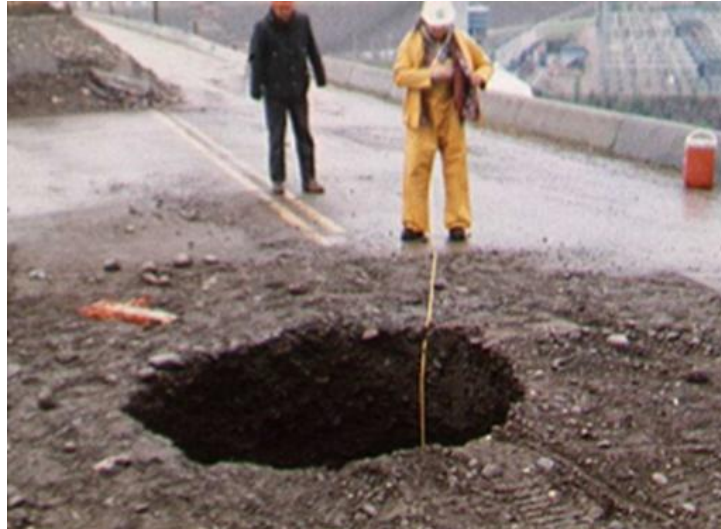
Figure 11.2.5.5-2. Sinkhole at W. A. C. Bennett Dam believed to be due to inadequate compaction of embankment materials near and around instrumentation installations.
